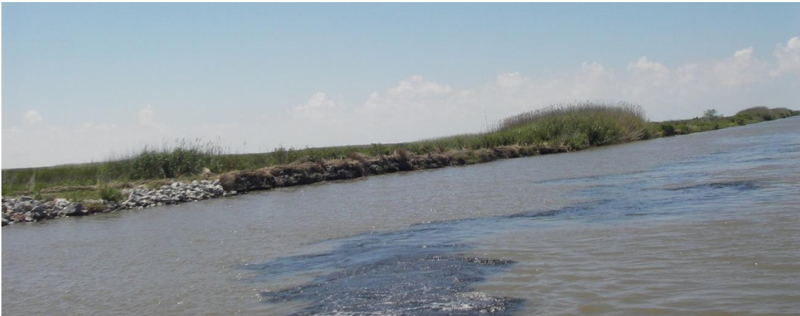
Photo No. 6 , MC Cell No. 1, Plug Tie-In (TV-14 Project- End of East West Canal - Looking SouthEast)
