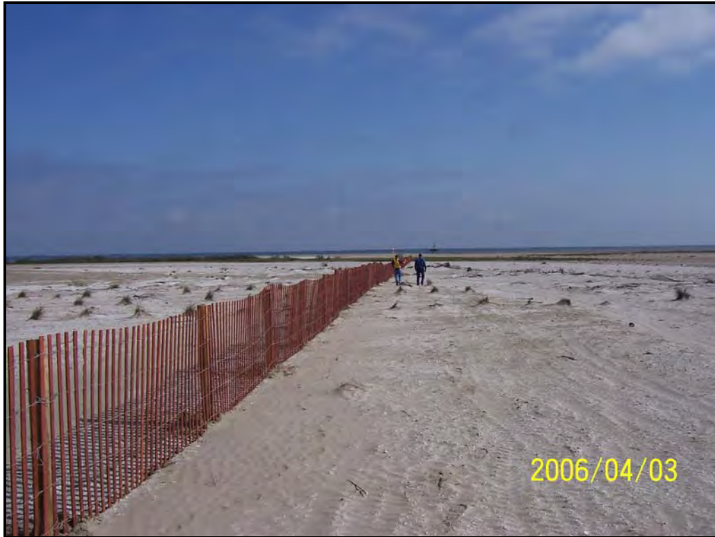
Photo 7. View of new fence at east end of dune platform looking northeast.
