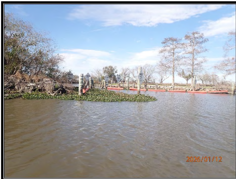
Photo No.2 – view of timber signage and floating debris barrier at Brady Canal Structure.
