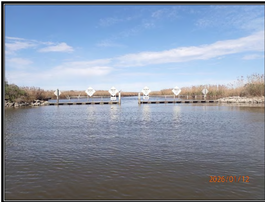
Photo No.8 – overall view of the weir structure and signage with at Site No.4.
