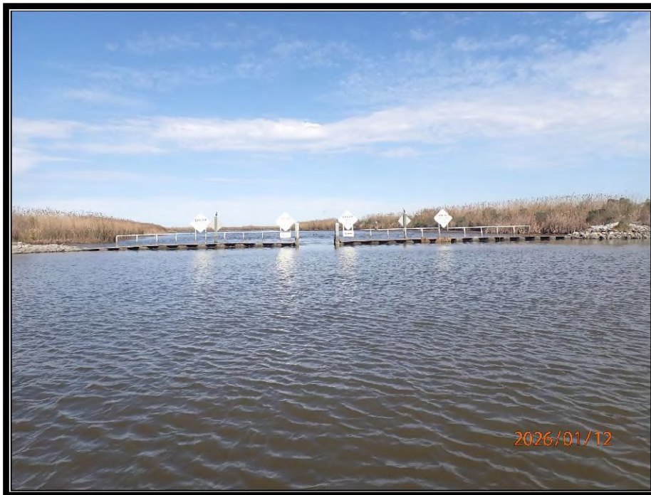
Photo No.10 – overall view of weir structure and signage at Site No.5.
