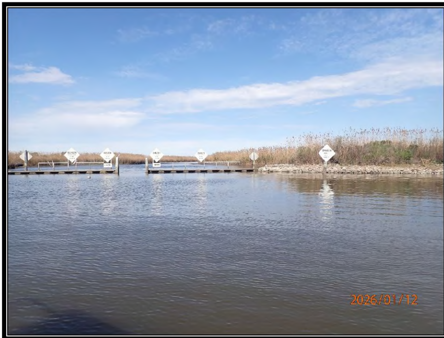
Photo No.6 – view of weir structure at Site 4 along Bayou Decade near Lost Lake and rock tie-in to steel sheet pile on the south side of the structure.
