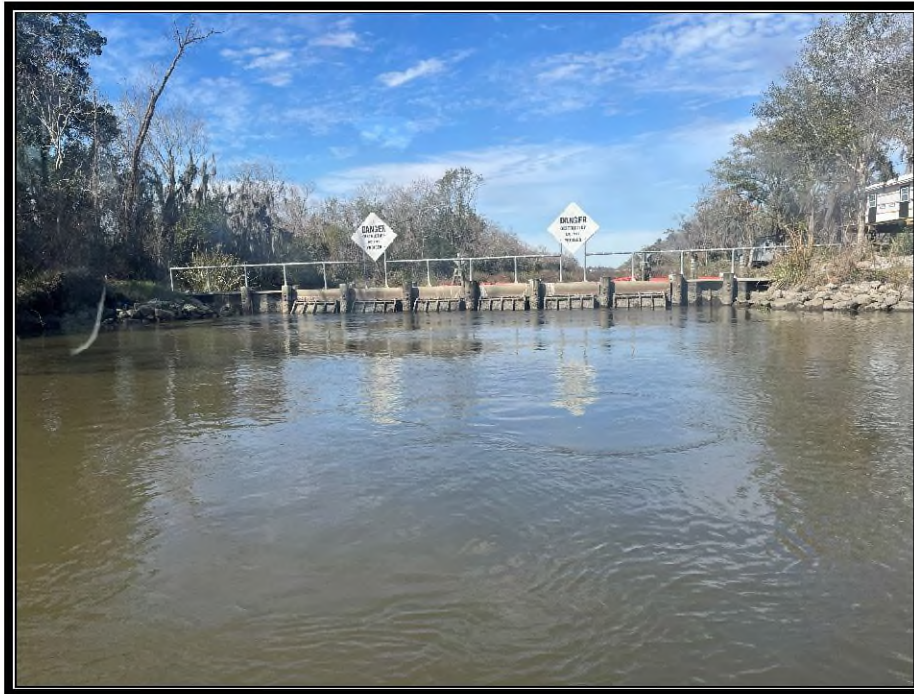
Photo No.5 – view of weir flap gates on the structure along Superior Canal.
