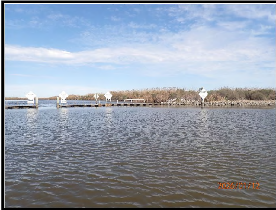
Photo No.11 – Rock dike tie-in to the steel bulkhead weir on the north side of the structure at Site No.5.
