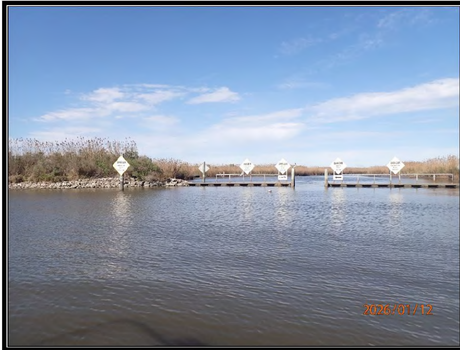
Photo No.7 – Rock dike tie-in to the steel bulkhead of Site No.4 and signage.
