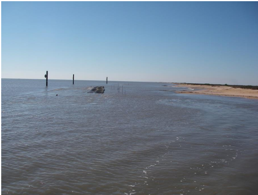
Figure A-12. Standard-Weight Oysterbreak in Foreground and OysterKrete Oysterbreak in Background between the two poles on March 12, 2013 as Tide rises; notice that all of OysterKrete Oysterbreak is already under water. Small pvc poles behind Oysterbreaks are Locations for Experimental Cages with Cylinders and Tiles. Photo by Tommy McGinnis.
