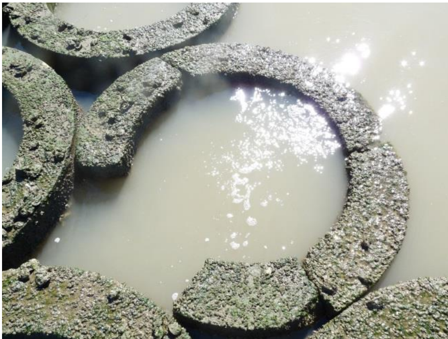
Figure A-14. Standard-Weight Oysterbreak Top-Tier Ring on West end of Structure showing Stress Fracture on October 28, 2013.
