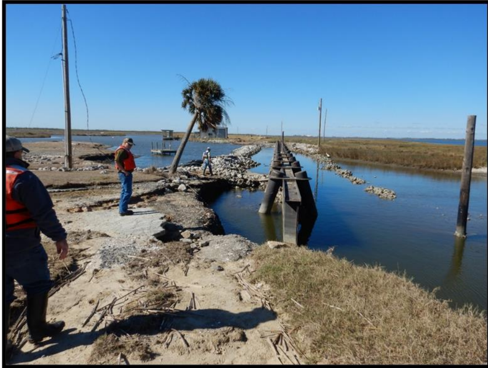
Figure 16. No Name Bayou Levee Breach Structure - Scouring Around Structure, Post-Hurricane Laura
