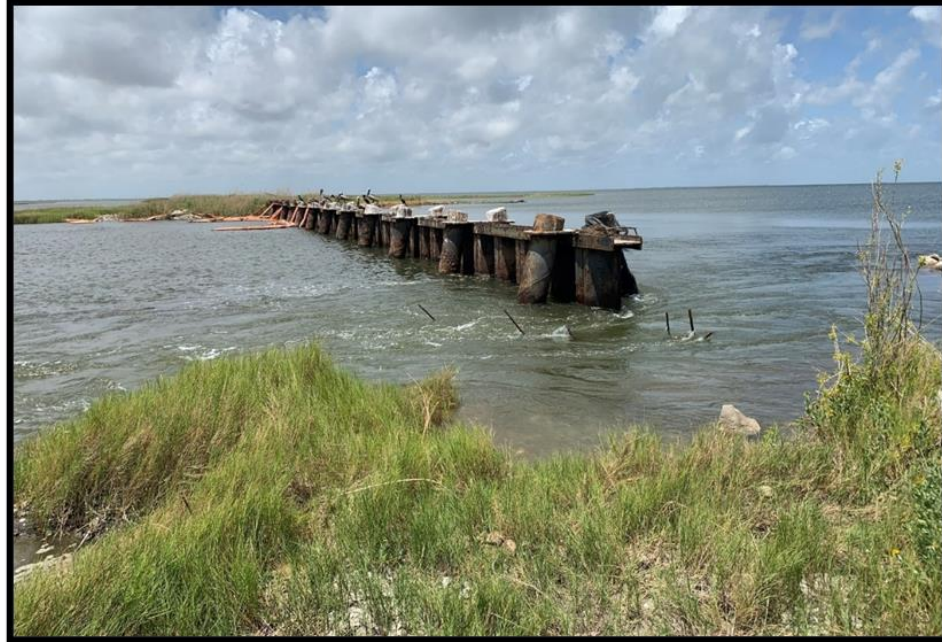
Figure 14. Lambert Bayou Levee Breach Structure - Overview of Scouring on North East End, Post-Hurricane Laura
