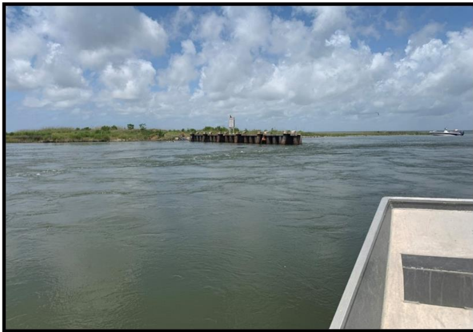
Figure 13. Grand Bayou Levee Breach Structure - Overview of Scouring on North End, Post-Hurricane Laura
