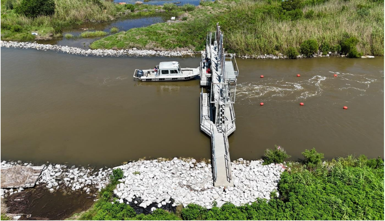
Figure 21. Grand Bayou Water Control Structure, Post-Construction
