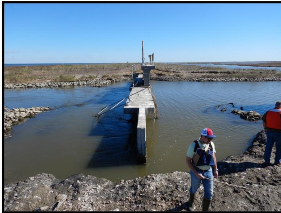
Figure 15. No Name Bayou Water Control Structure - Scouring of Tie-Ins, Post-Hurricane Laura
