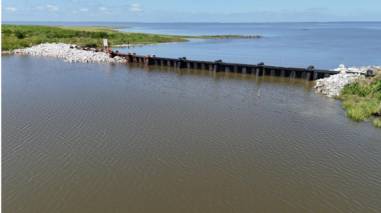
Figure 22. Grand Bayou Levee Breach Structure, Post-Construction
