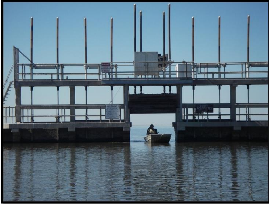
Figure 4. Grand Bayou Water Control Structure, Pre-Hurricane Laura
