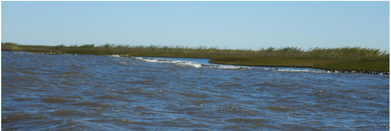
Photo No. 8 – Sabine Lake Foreshore Rock Dike, Low area of Rock
