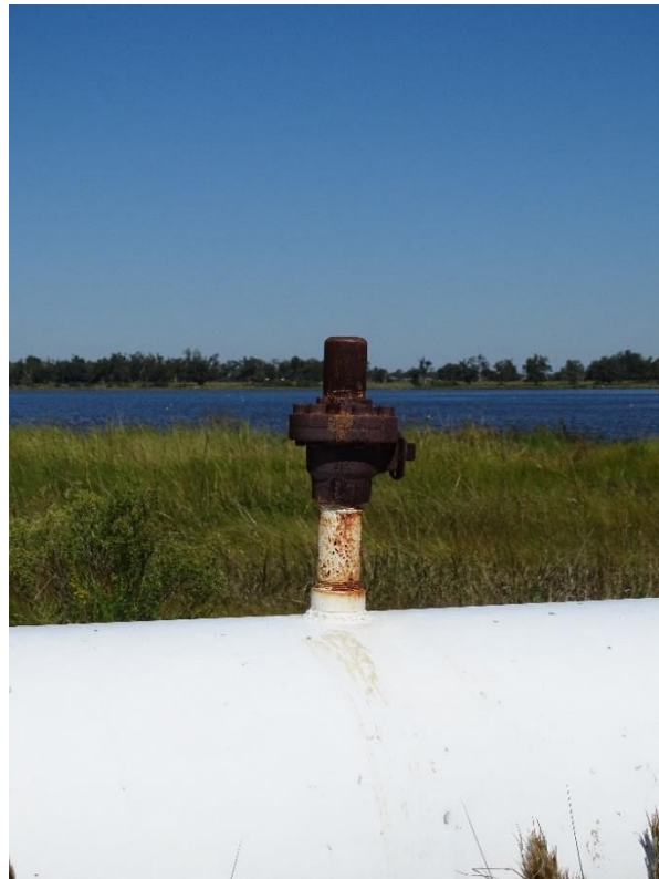
Photo No. 22, West Blind Flange and Riser, Vent Looking South
