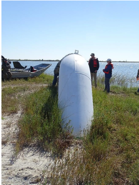
Photo No. 3, East end blind flange and riser (looking East)
