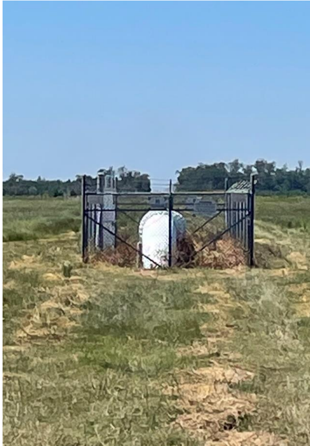
Photo No. 11, East Booster Station – looking west
