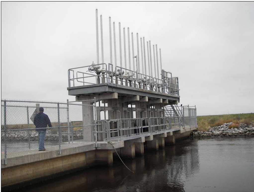
Photo No. 6, West Cove Canal from Hwy 27 side – gates being exercised and in open position
