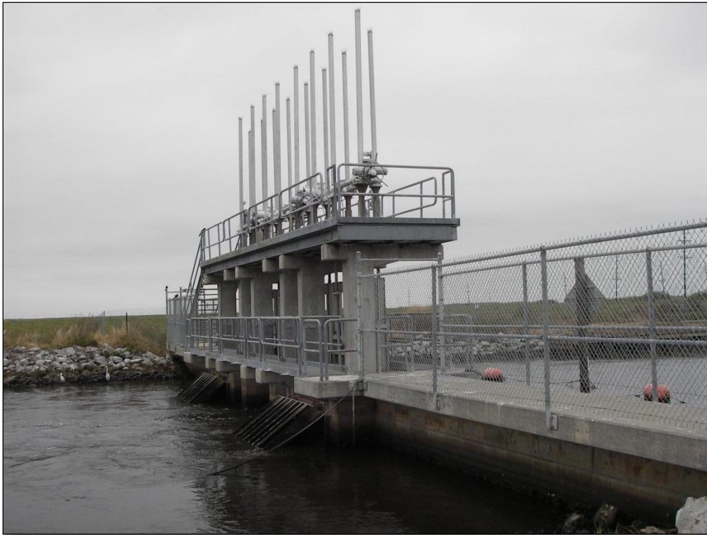
Photo No. 5, West Cove Canal Calcasieu Lake side of structure with flapgate flapping
