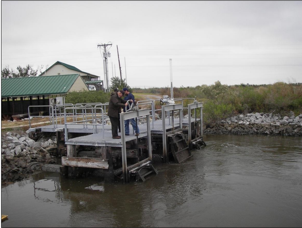
Photo No. 3, Headquarters Structure with outside flapgates flapping
