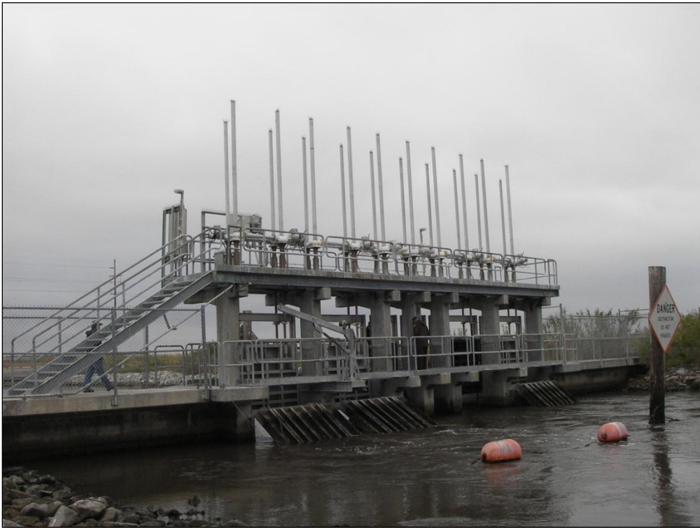
Photo No. 2 , Hog Island Gully Structure from the Calcasieu Lake side– gates being exercised and in open position
