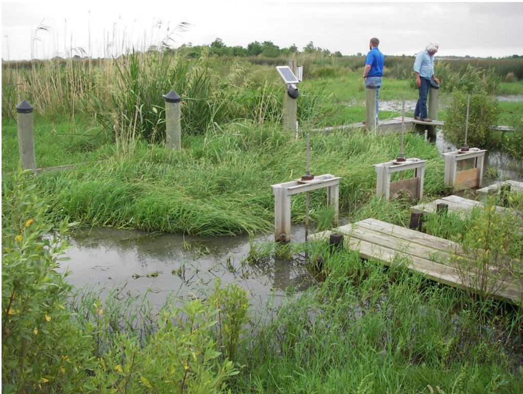
Photo No. 2, Structure No.1, Inlet Side- Inlet Channel, Hyacinth Fence and Operations Equipment
