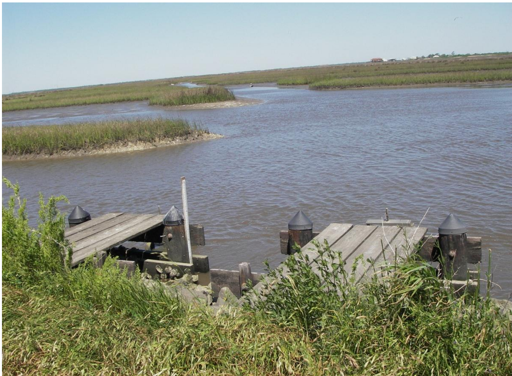
Photo No. 6, Structure No. 12, Outlet Side- Water Flowing Out to Lakeside (April 2014)
