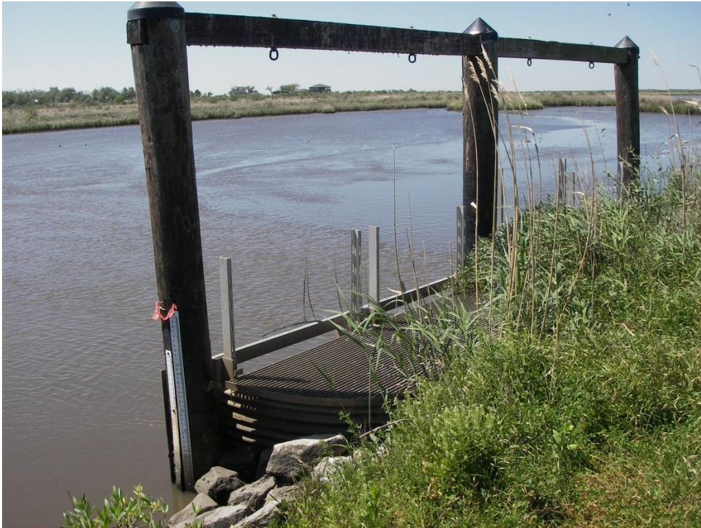
Photo No. 5, Structure No. 12, Inlet Side- New Staff Gauge (April 2014)
