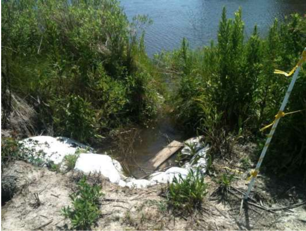
Photo #3 – WCS Berm Erosion Above Culverts
