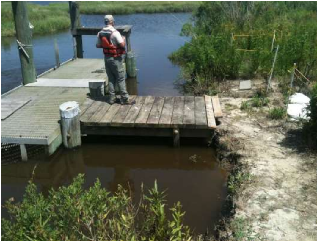
Photo #4 – Erosion on Marsh Side of WCS Berm
