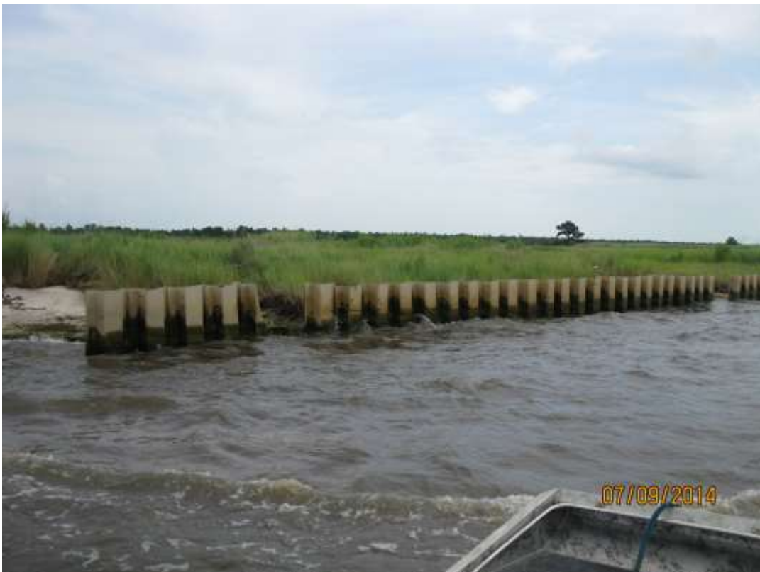
Area D – Apparent vandalism; sheet piles appear to have been cut
