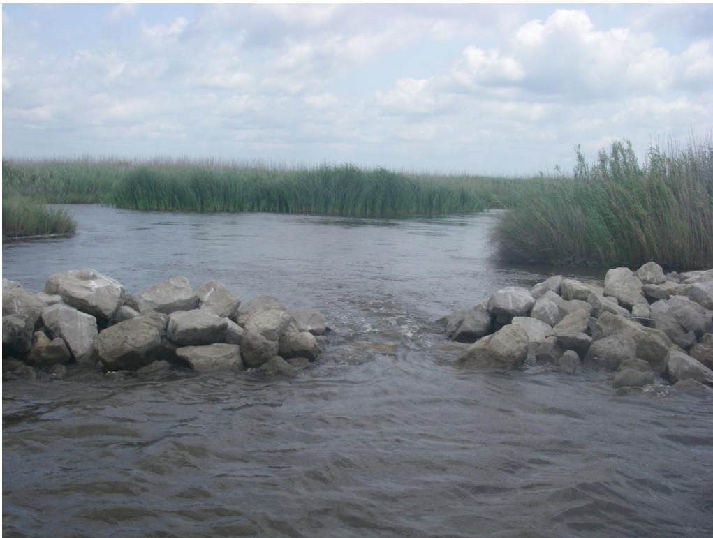
Photo No. 4, Water Flow through Displaced Rock Dike, Water Flow Channeling into Marsh
