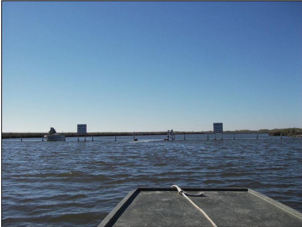
Photo 2 , Grand Bayou Weir, view showing missing boat guides.
