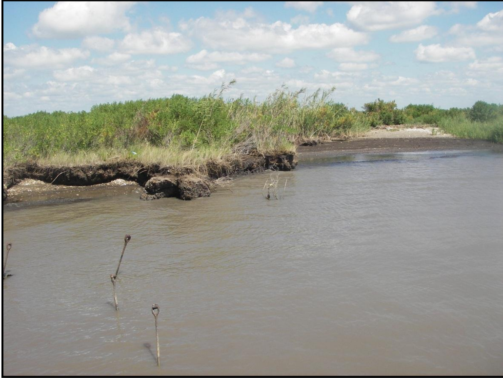
Photo 3: Area 2- Close Up View of Erosion on East Side of Concrete Mats
