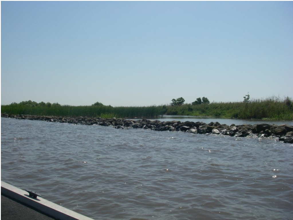
Photo No. 2, Vegetation and Rock Dike on East Shoreline of Grand Lake
