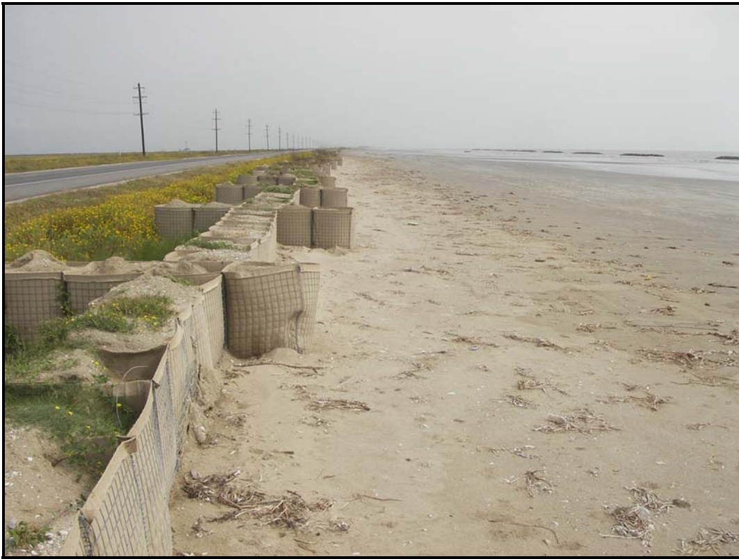
Photo No. 5, HESCO Baskets located along the eastern portion of the project area.
