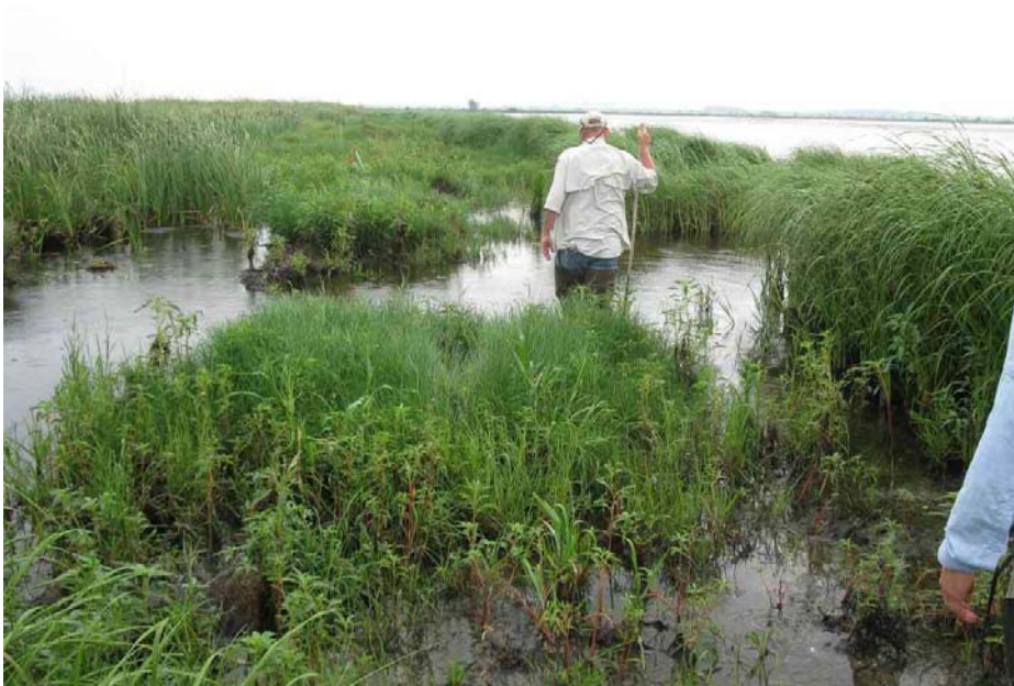
Photo # 2 – Containment Dike Gap - Marsh Creation Area 2
