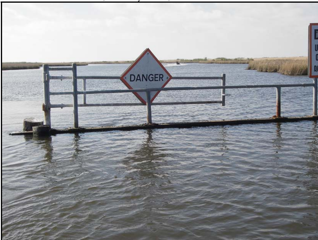
Photo 2 , Grand Bayou Weir, close up view showing missing boat guide west side.
