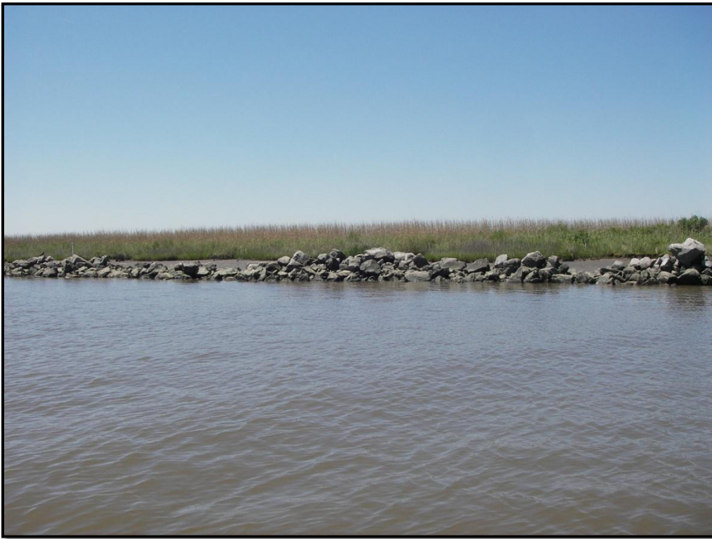
Photo No. 3, View of typical low area showing stable bank behind dike as well as low sections of dike
