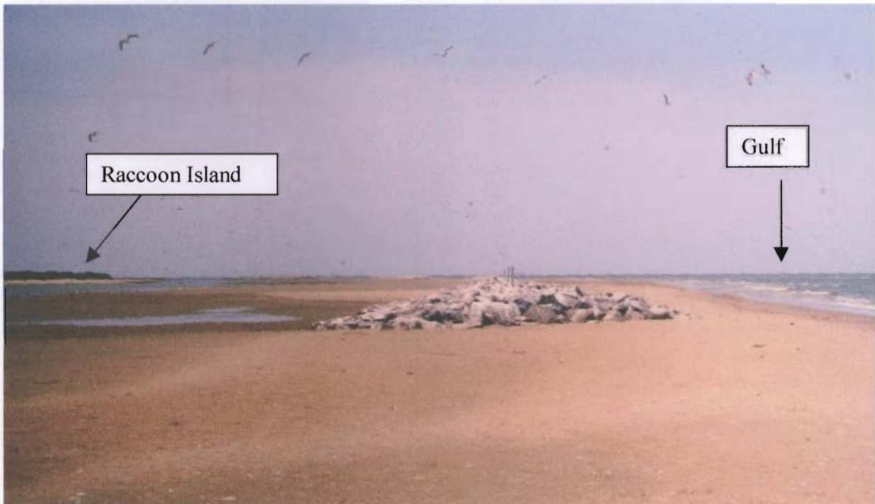
Plate 3. The breakwaters #6, #5, #4, and #3 were surrounded by an emerged sand body both landward and seaward and the structures were not directly exposed to wave action. Photograph looking east, July 31, 1998.
