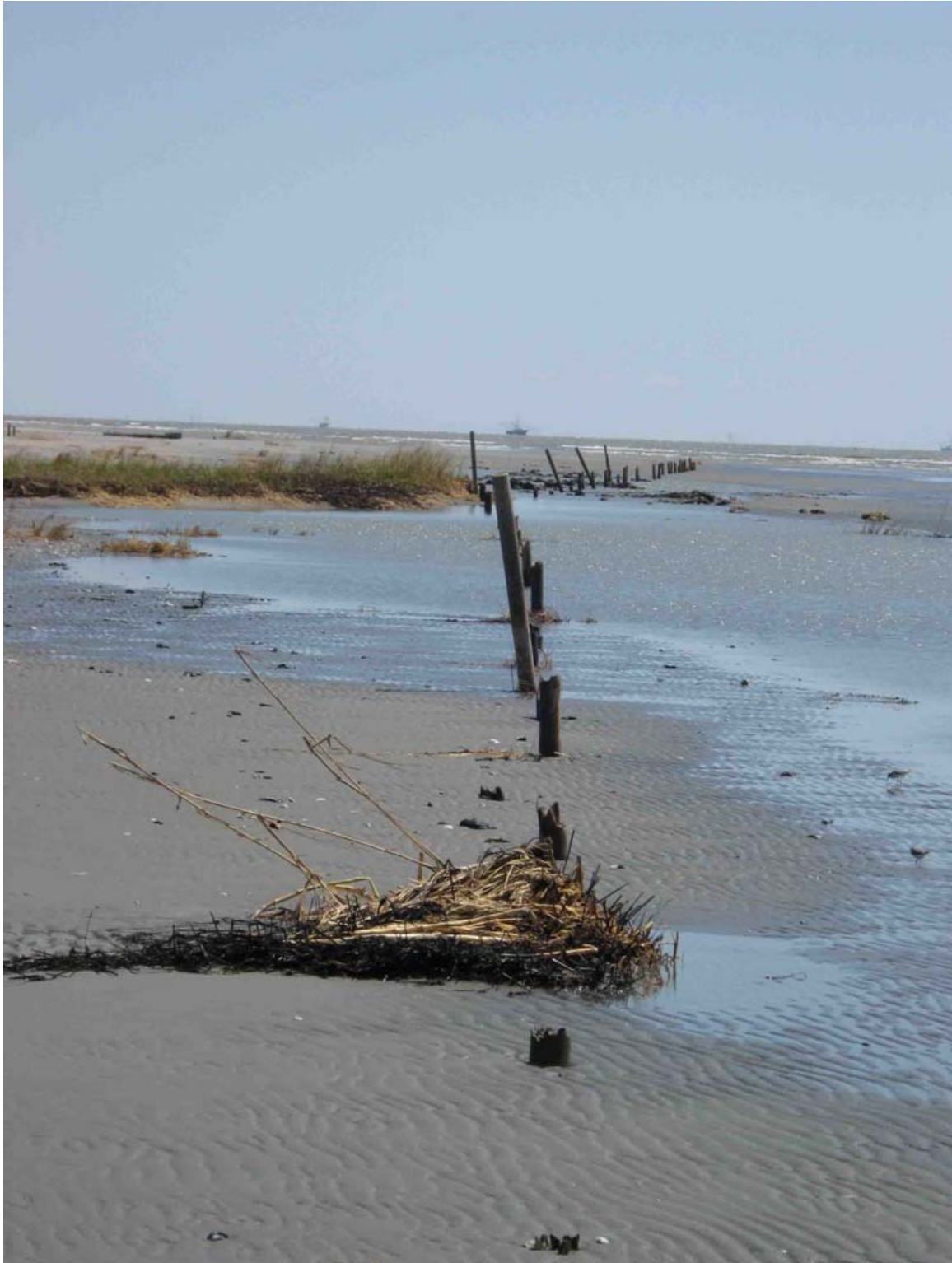
Photo #1 –Damage to Sand Fence (now in surf line).
