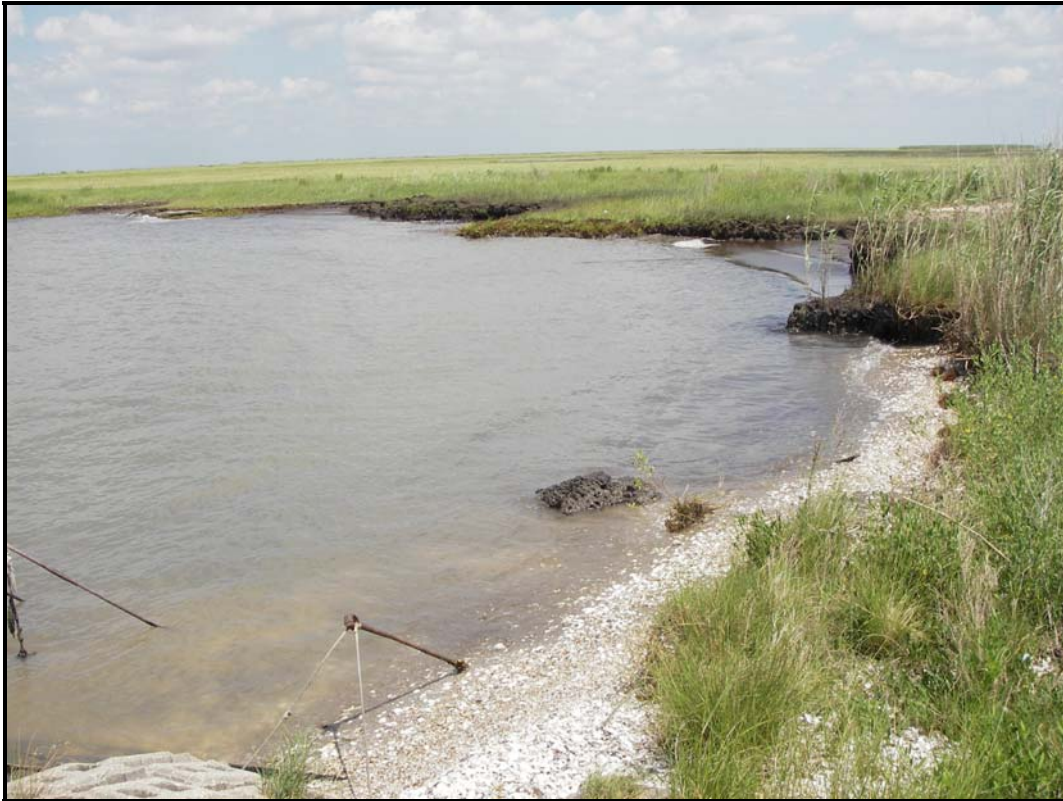
Photo 3, Area 2, Close up view of erosion on west side of concrete mats.
