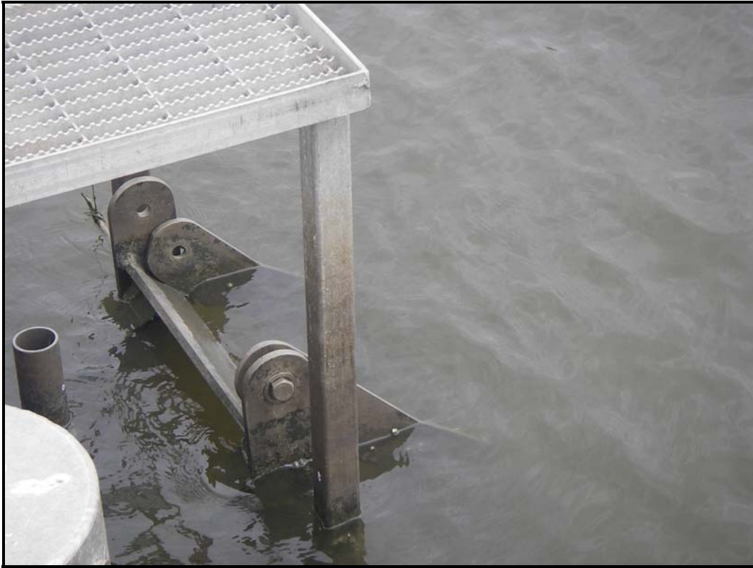
Photo 5 , View showing missing hardware.
