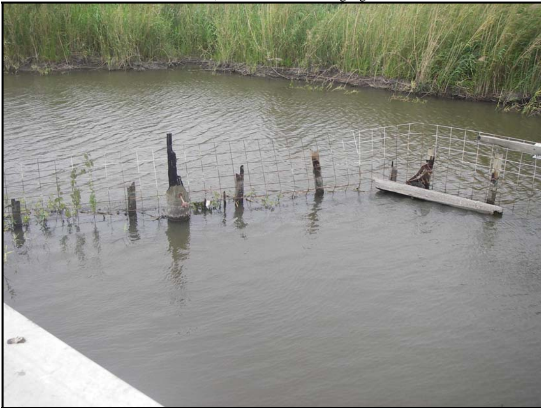
Photo 2 , Inlet side showing burn damage to hyacinth fence.
