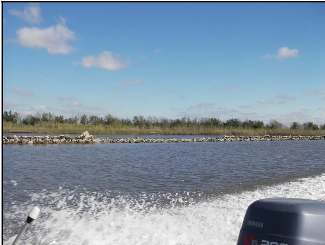
Photo 2 —Area of dike slightly low in elevation.
