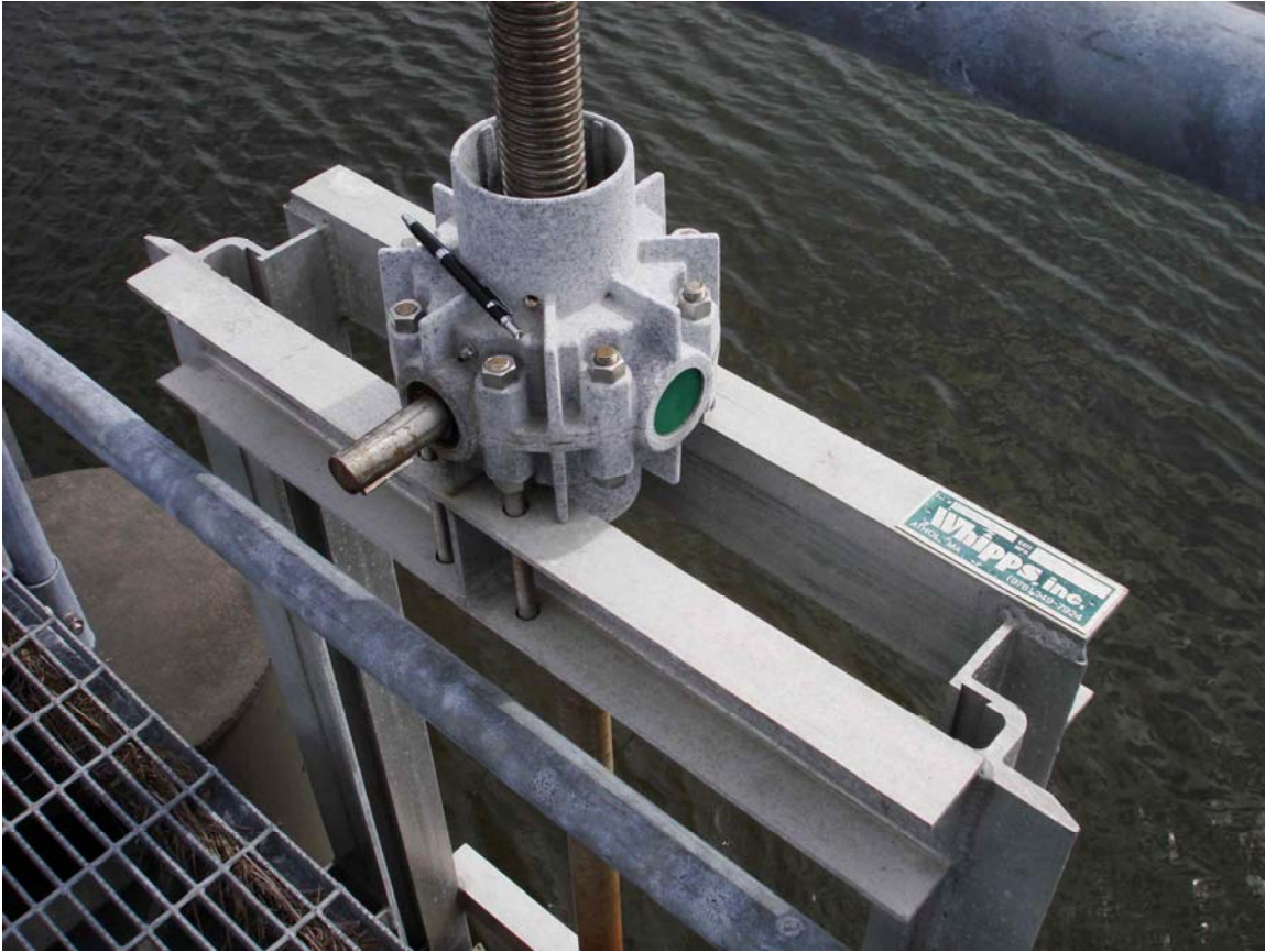
Photo #2 – Fish Gate Operator. The stem protective cover is missing and needs to be replaced on both fish gates and all three flap/slucice gates. A locking mechanism should be installed to prevent unauthorized operation of the gates.
