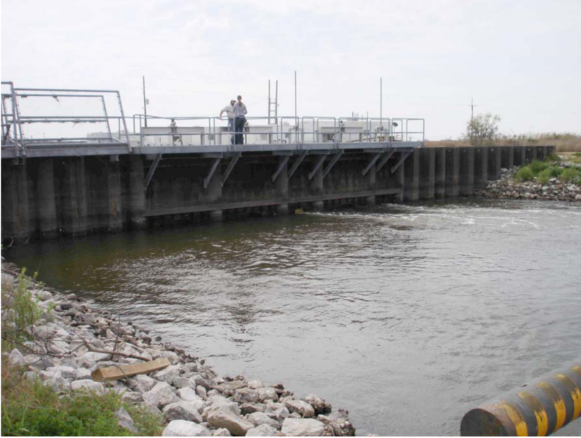
Photo #1 – Water Control Structure. Standing on the East bank looking south. Note the damage to the railing and fencing.
