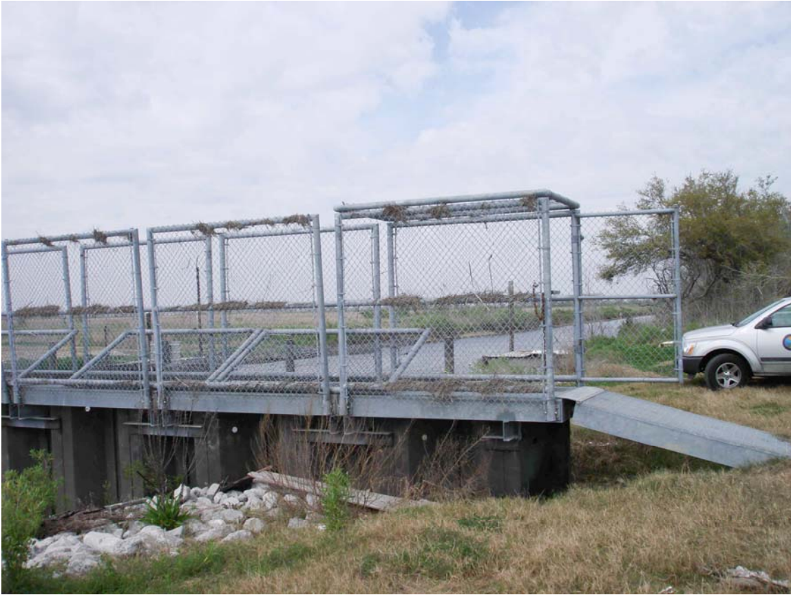
Photo #3 – Ramp and Entry. Standing on the East bank looking north. Note the damage to the railing and fencing and the scour around the end of the sheet pile wall.
