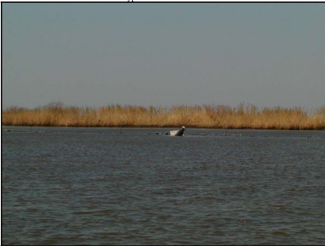
Photo 10 — damaged warning sign on School Bus Bayou dike
