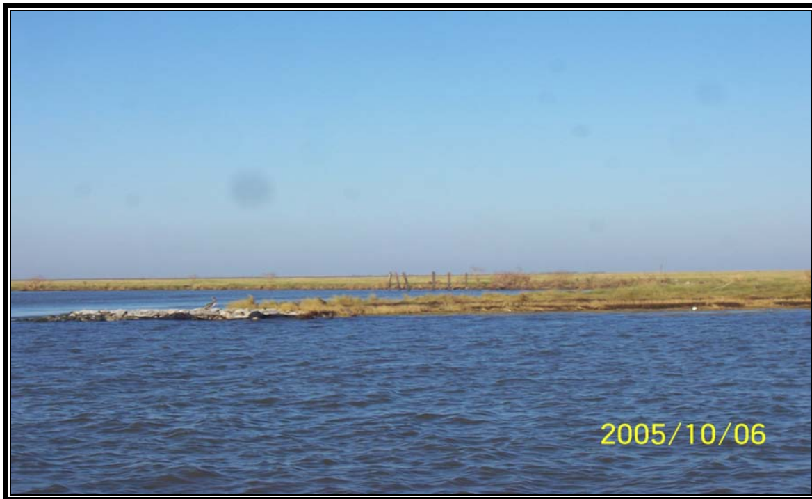
TE-26 – Structure No.3 – photo showing erosion along the shoreline on the north side of structure looking southwest.
