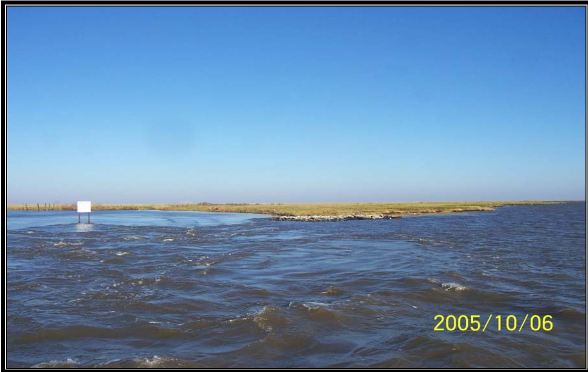
TE-26 – Structure No.3 – photo showing erosion along the shoreline north of rock rip rap weir looking west.
