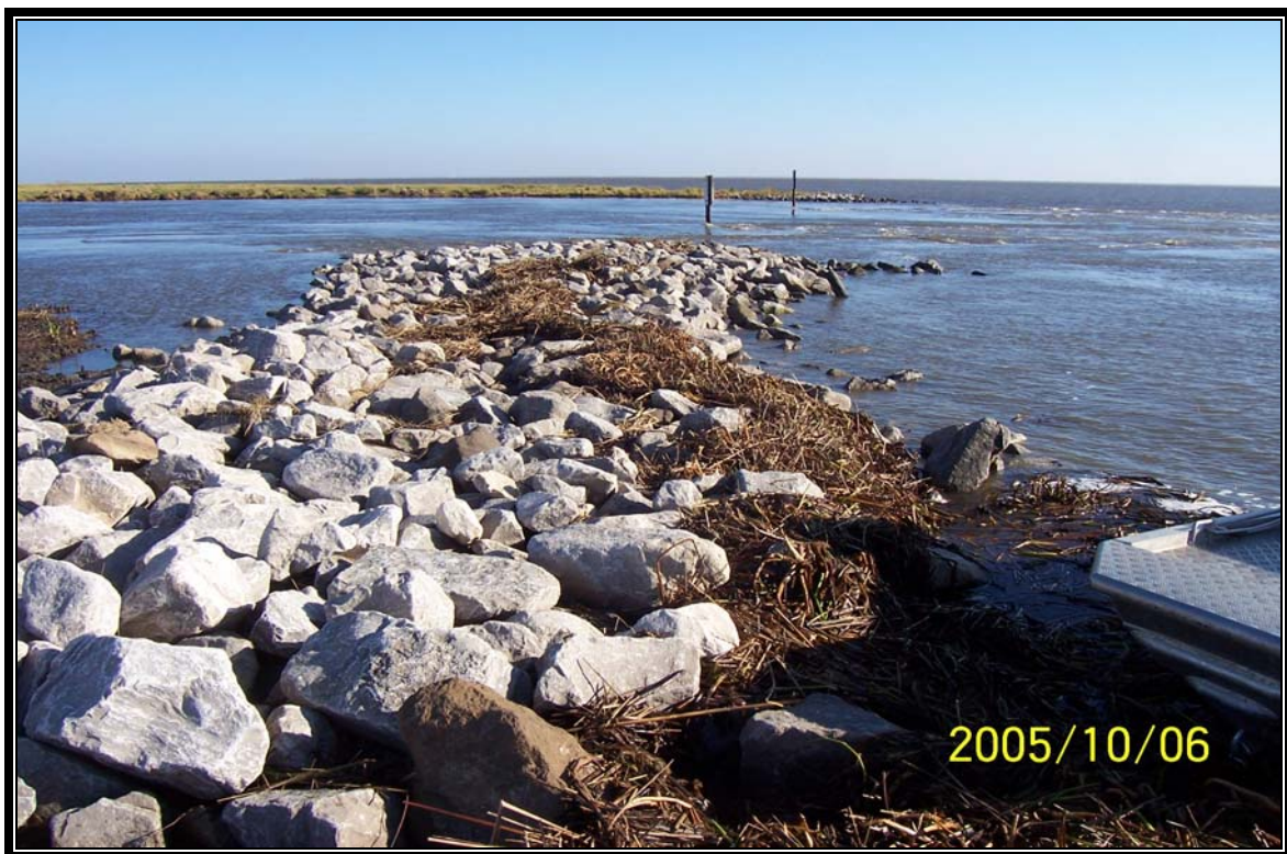
TE-26 – Structure No.3 – rock riprap weir with boat bay located along the southwest bank of Four League Bay looking north.
