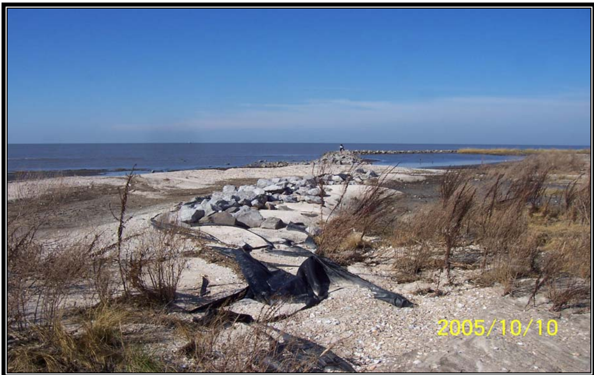
TE-22 –Photo of displaced rock rip rap along rock dike located adjacent to the east end of Mobile Canal along the Gulf of Mexico.
