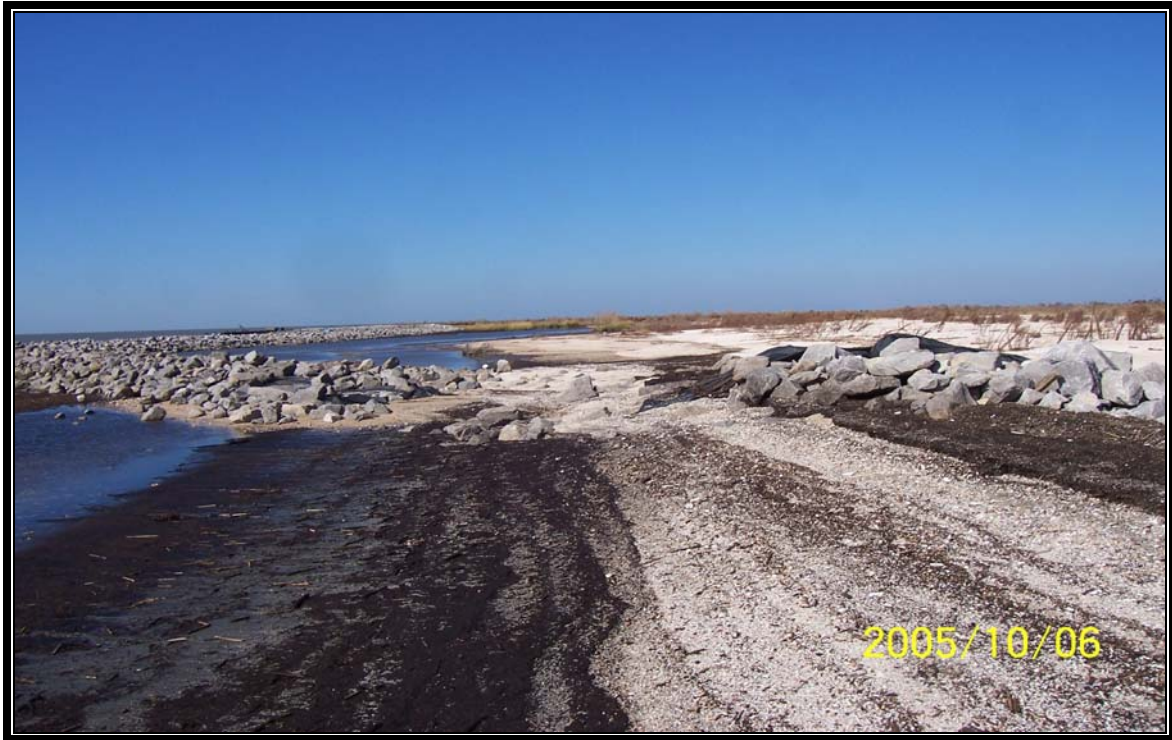
TE-22 –Photo of displaced rock rip rap along rock dike located on the east side of the steel sheetpile bulkhead at the end of Transco Canal along the Gulf of Mexico.
