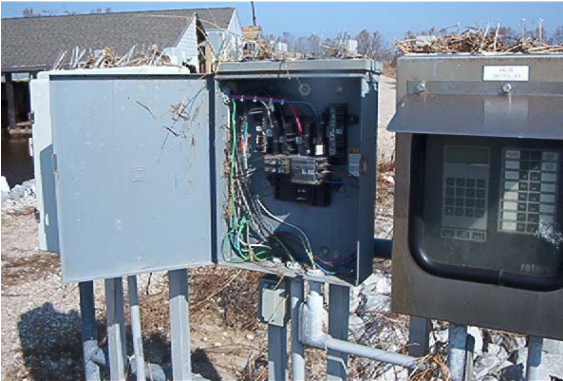
Photo 4, Grass and Water Inside Panel Box Headquarters' Canal Structure
