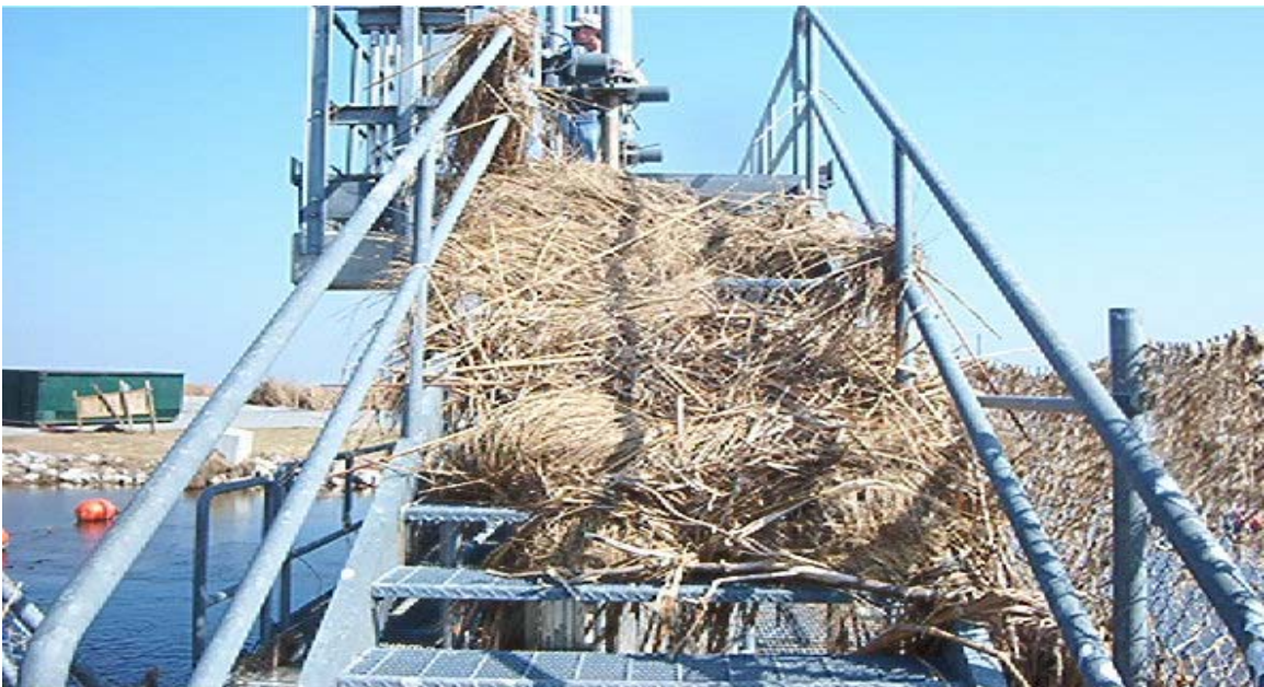
Photo 8, Storm Surge Topped The Top Platform At West Cove Canal Structure
