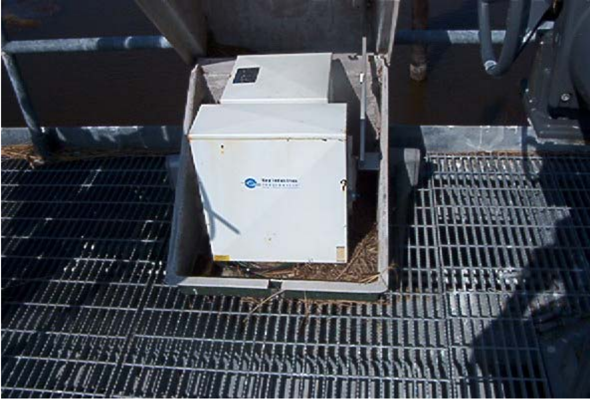
Photo 7, Grass And Debris Inside Variable Frequency Drive Enclosure West Cove Canal Structure
