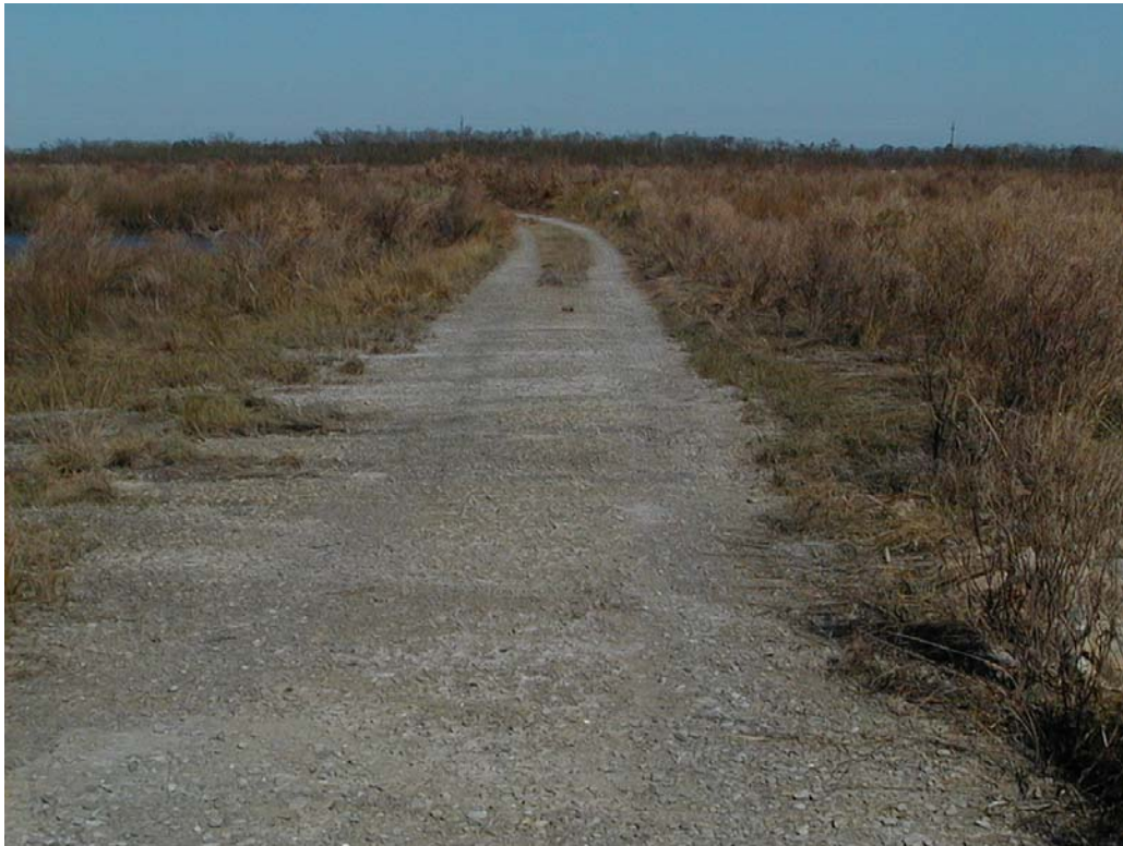
Photo 6, View of access road just east of structure No. 12 showing washout of roadway.
