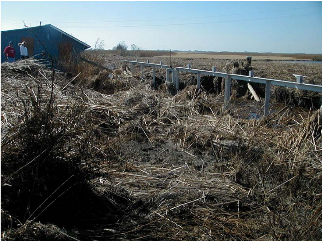
Photo 2, Inlet side showing hyacinth fence in background covered with debris, as well as embankment of structure.
