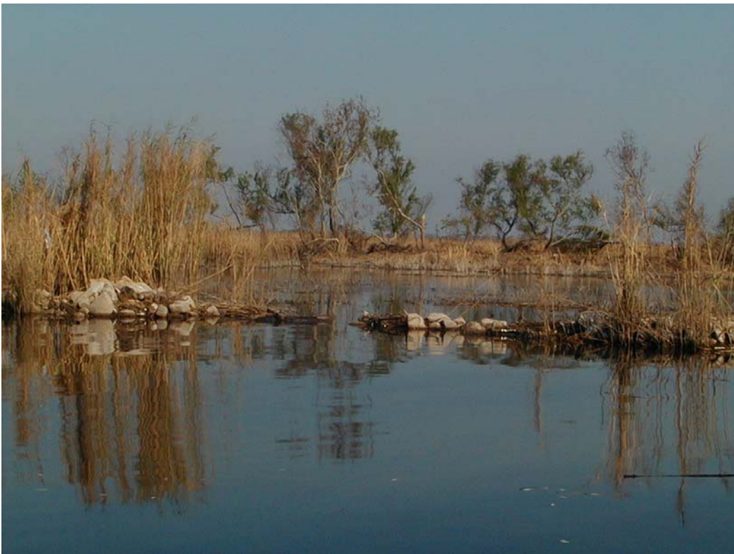
Photo 4, Low area/displaced rock area along dike.
