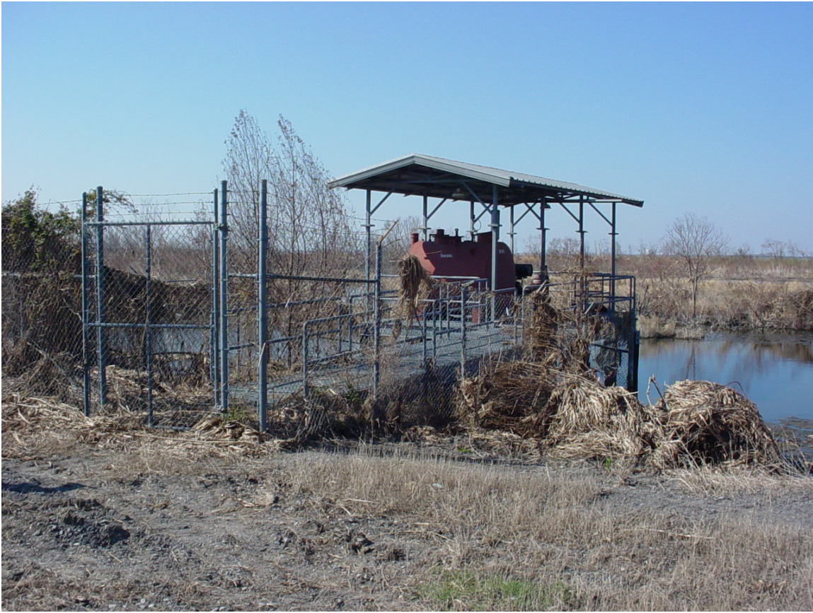
Photo #1 – Pump #6. Notice the debris on the fencing for the walkway showing that the water was at least that high at one point.
