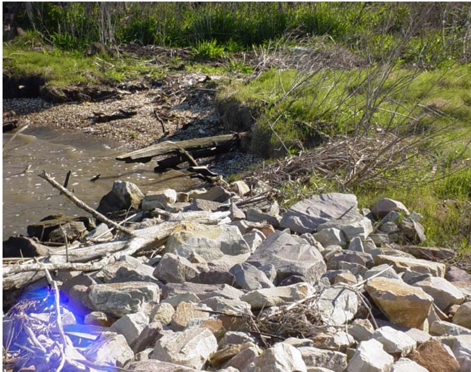
Photo #6 Erosion at west end on CU3.
