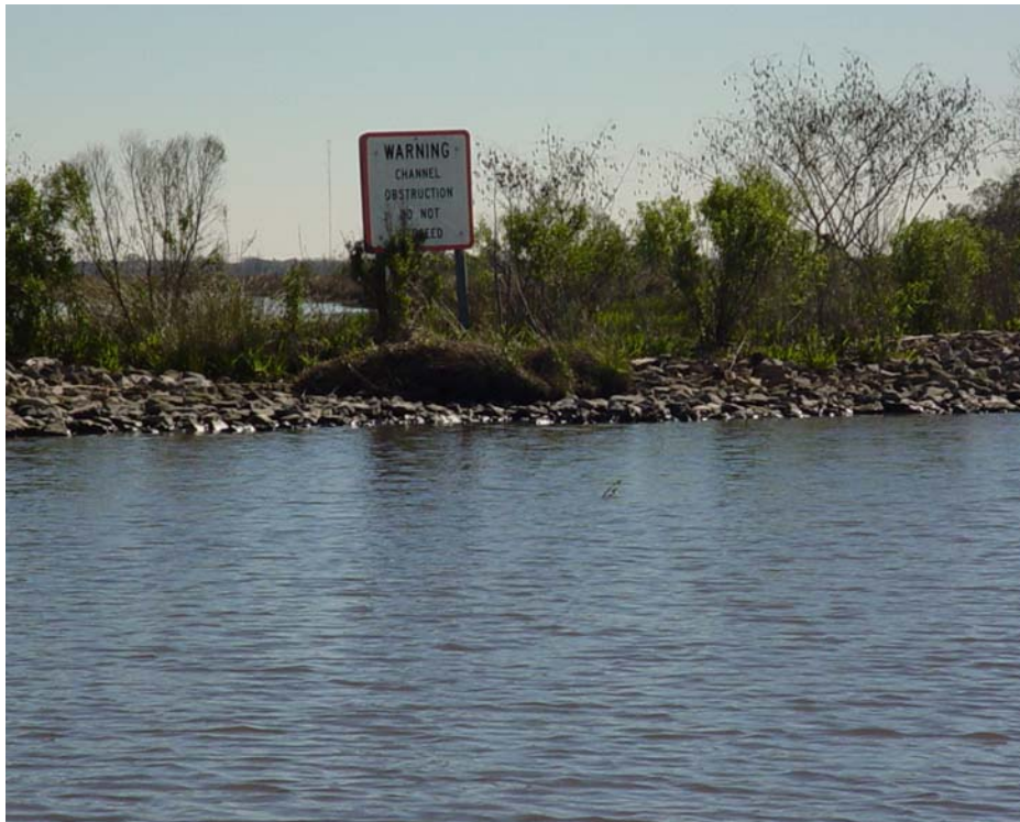
Photo #4 Low spot on Structure #17
