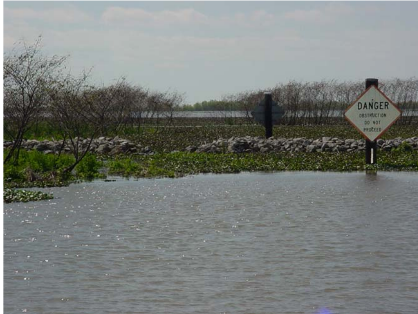
Photo # 5 Site 32 (view 1) This structure was opened to the waterline by vandals and was partially repaired by the 2003 inspection team. Destruction of the west lake rim of Lake Lery by the storm, now makes this closure irrelevant.
