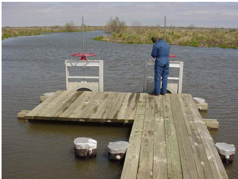
Photo # 20 Site 60 (View 2) Structure is clear of all storm debris. The blockage of the culverts due to storm debris has been cleared. Some flow was visible through the culverts.
