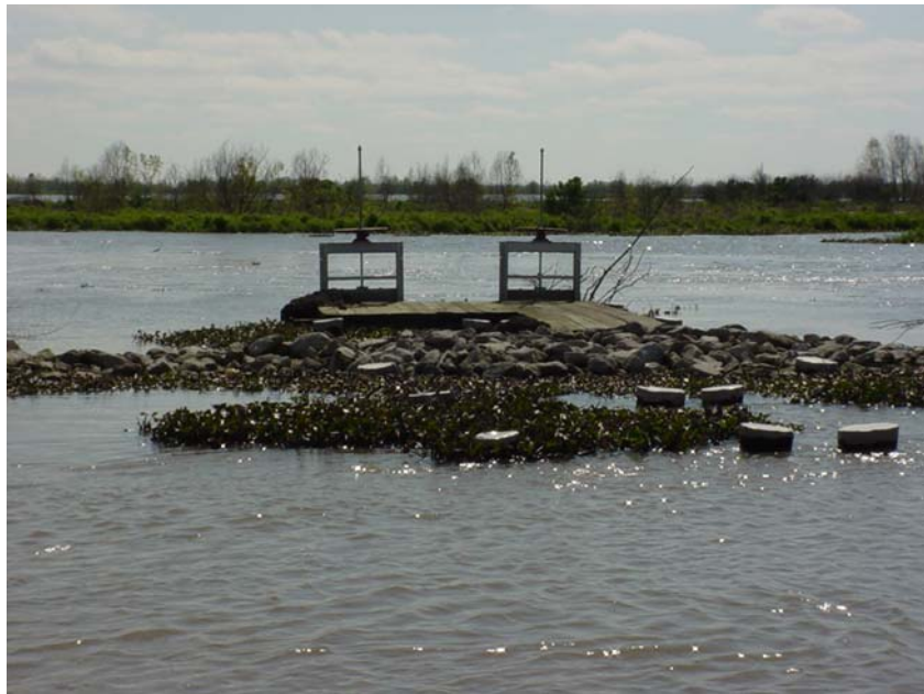
Photo # 9 Site 52 (view 1) Some storm debris remains on the inside of the culverts. A tree stump ball is blocking the north culvert opening on the inside. Slight erosion was evident on both sides of the rock plug where it ties into the earthen embankment.
