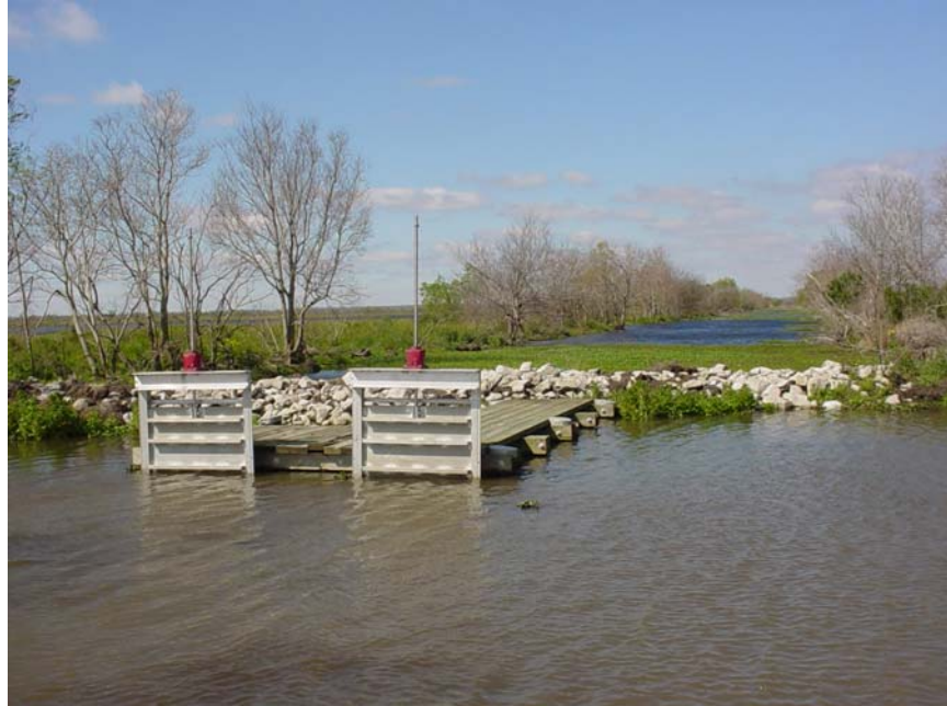
Photo # 11 Site 54. Structure is clear of storm debris. The blockage of the culverts from storm debris has been cleared. The flow-meter and all attachments on this structure that were destroyed by the storm will be replaced soon.
