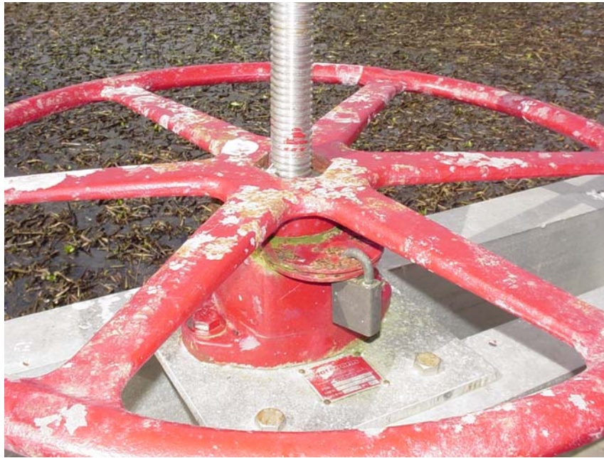
Photo # 1 Site 13 (view 1) Corrosion of locking plates caused them to separate making locking impossible.
