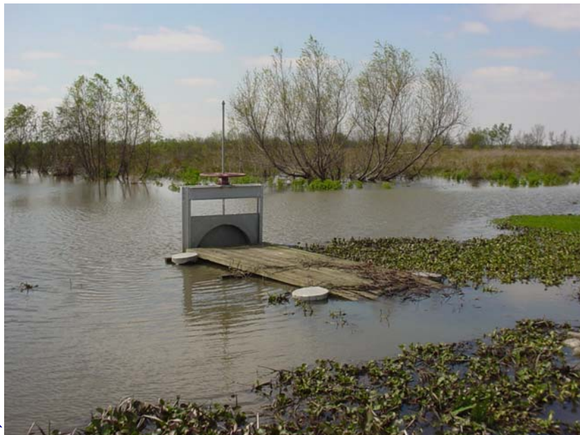
Photo # 8 Site 50 The extent of blockage of the culverts by storm debris is minimal. Slight erosion was evident on both sides of the rock plug where it ties into the earthen embankment. High flows such as this, allow water to flow around the structures to flood the marsh.
