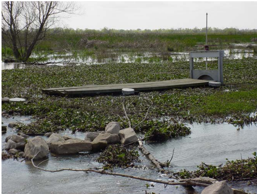
Photo # 2 Site 13 (view 2) The extent of blockage of the culvert due to storm debris is minimal. Note the high water stages in the inside, flowing out into Bayou Mandeville. Approximately ½ foot difference in water levels. (2007 Photo)
