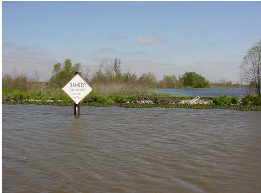
Photo #12 Site 56 The overall condition of the rock closure appears to be good. There is still much storm debris covering the closure. No noticeable subsidence has occurred since the last inspection.
