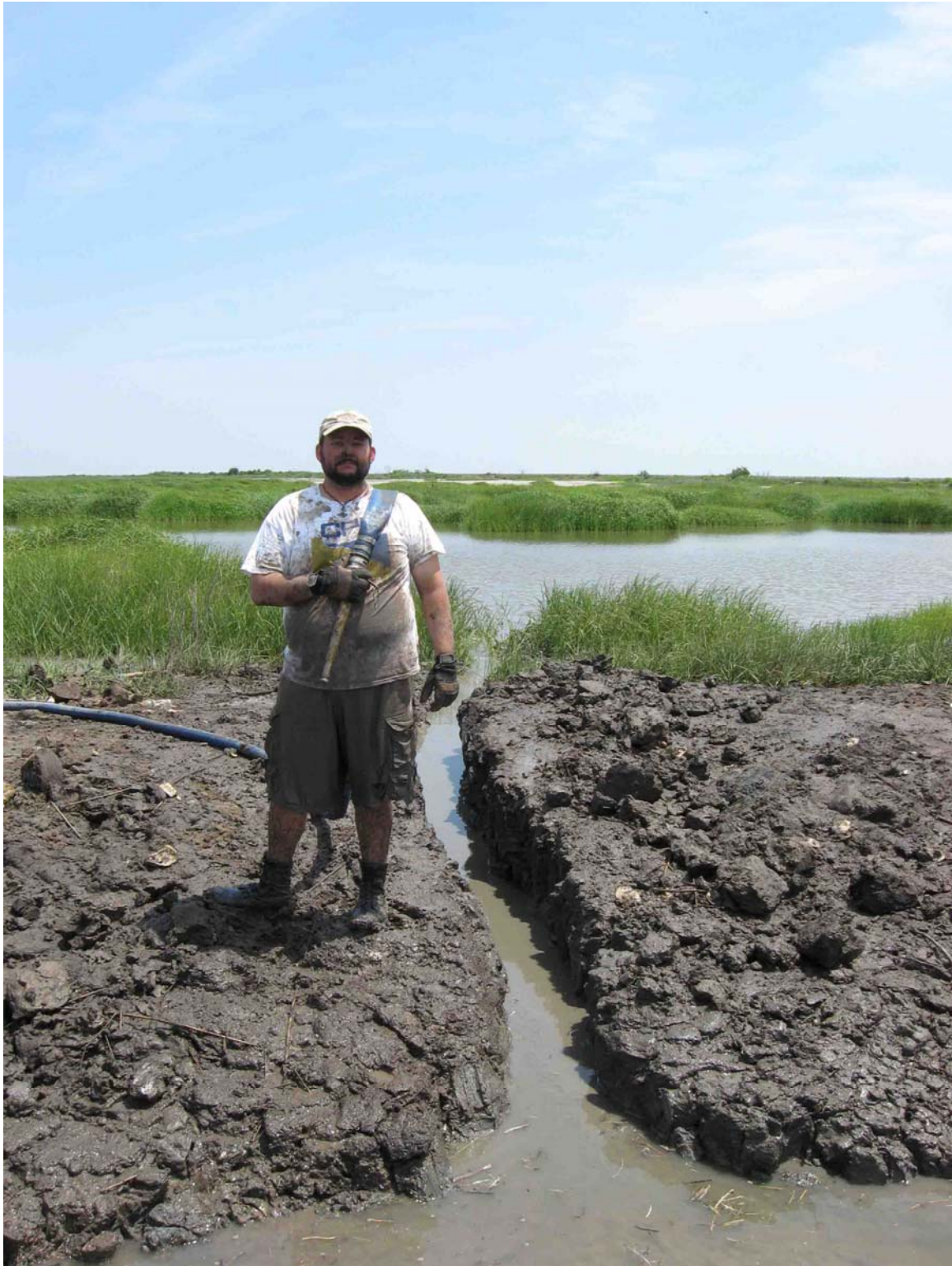
Photo #2 – Hydraulic Dike Gapping.
