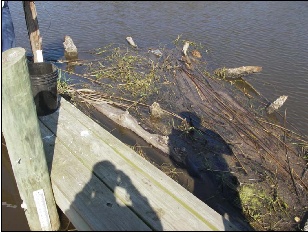
Photo No. 2, Structure No.1, trash along fence.
