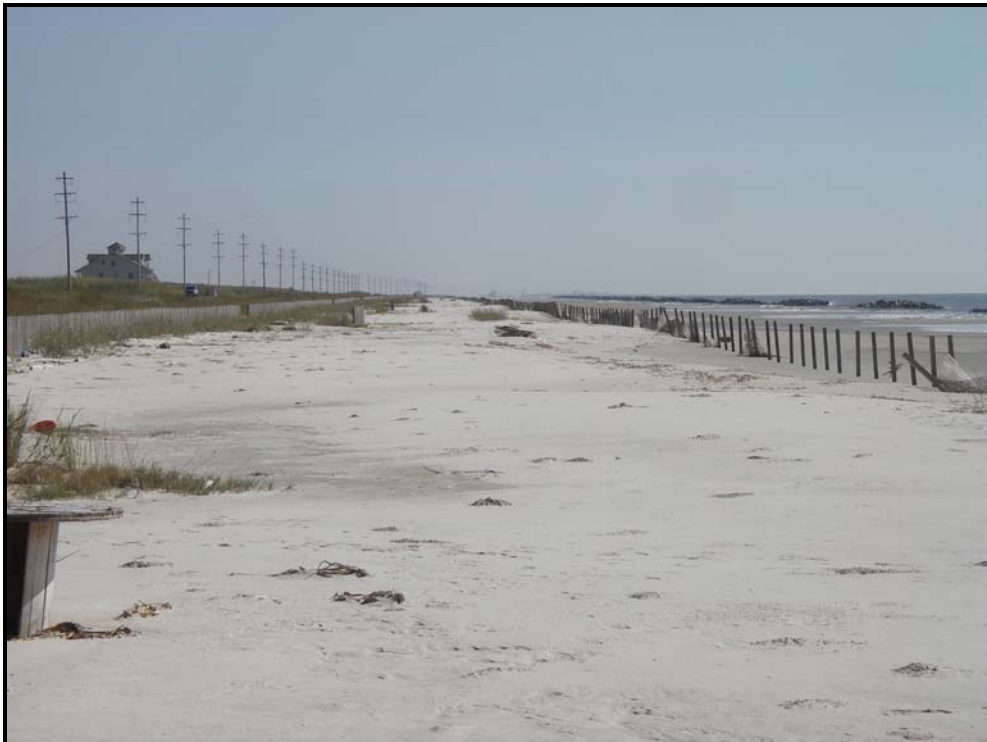
Photo 4, Secondary fence (from mid-project eastward) has sustained damage from high tide events. (10-30-2007)
