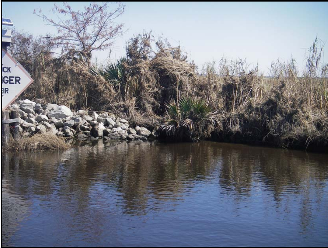
Photo 3 —erosion on SE end of Block's Creek Structure
