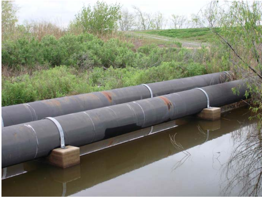
Photo #3 – Outflow. Discharge pipes from pump station to levee.
