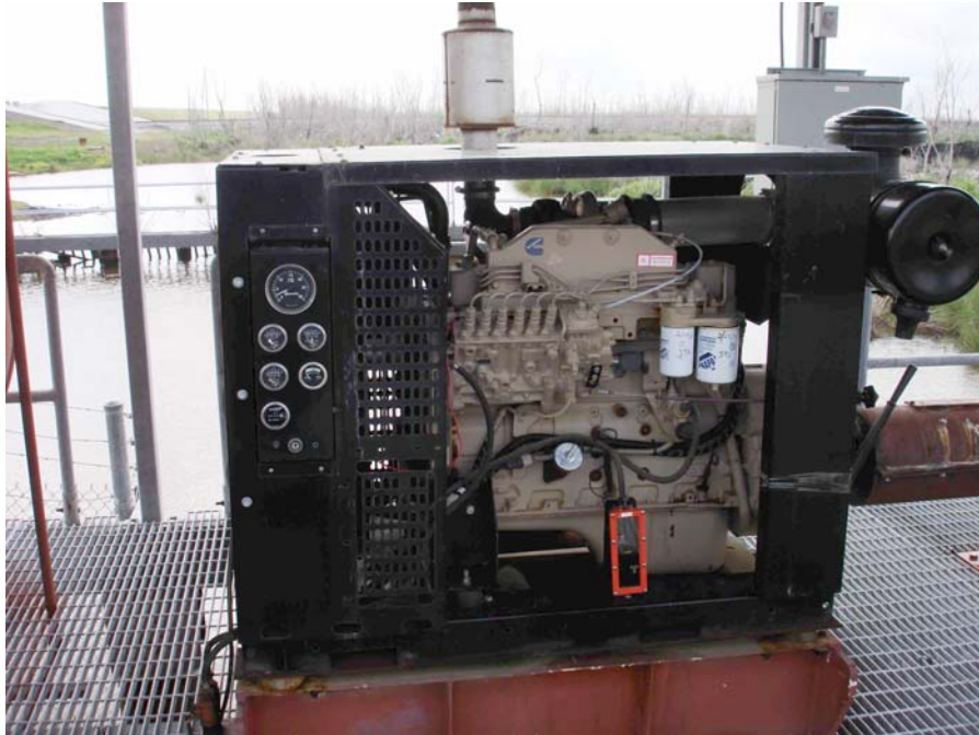
Photo #1 – CTU #5. New pump engine.
