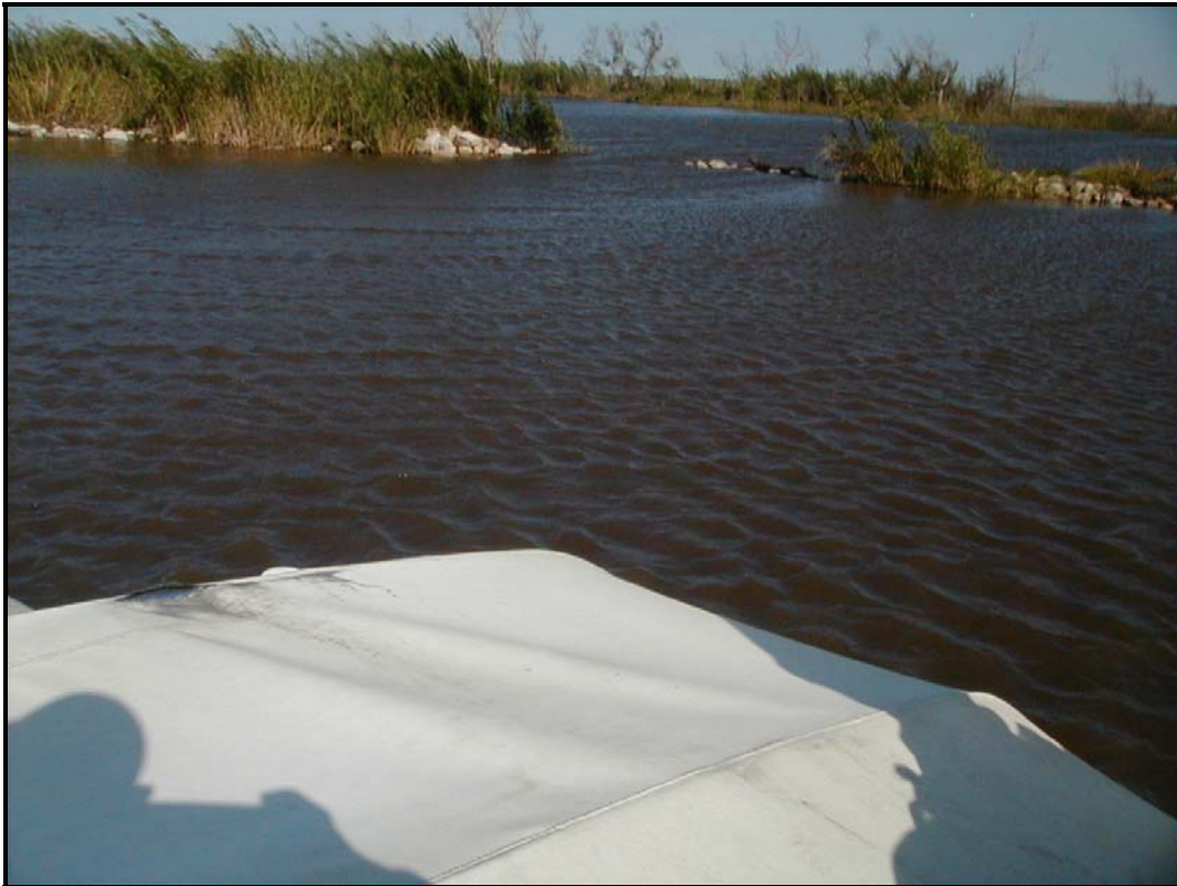
Photo 3, Low area/displaced rock area along dike.
