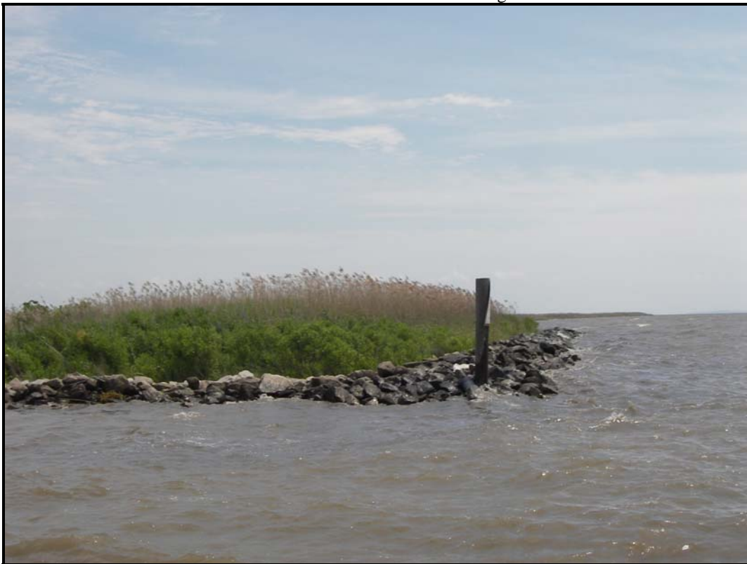
Photo 2 —south east side of Boston Canal at shoreline
