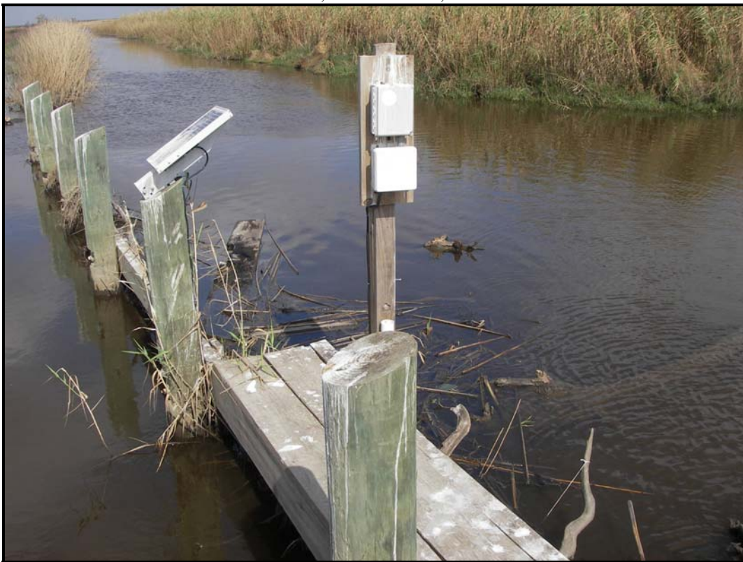
Photo No. 2, Structure No.1, trash along fence and operational sonde.
