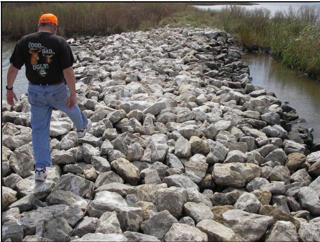
Photo No. 6, Structure No. 8, rock plug showing accretion occurring on lake side.
