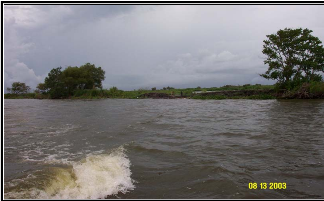
Breach 10 – photo of breach repair along the west bank of Jug Lake.
