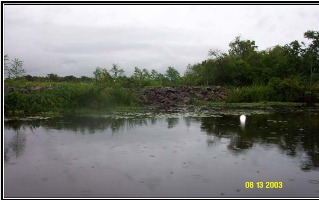
Breach 7 – Photo of rip-rap breach repair along oil field canal looking north.
