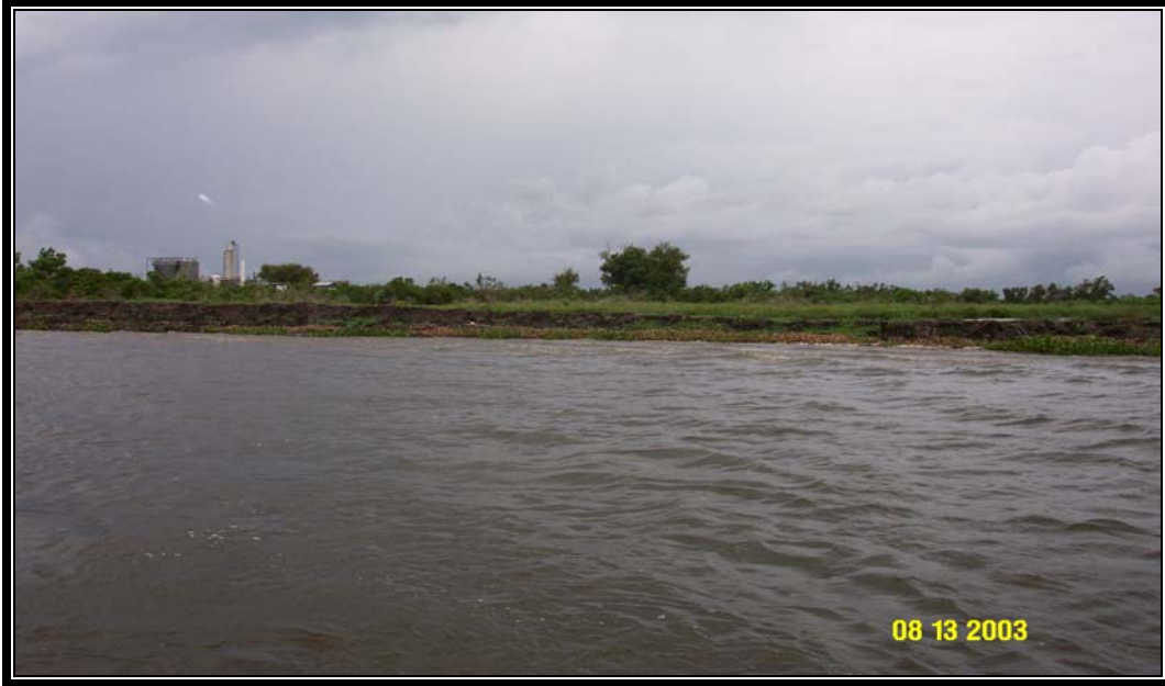
Breach 11 – photo of breach repair along the west bank of Jug Lake.
