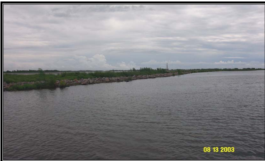
Breach 1 thru 4 – rock dike along Bayou Decade looking north.
