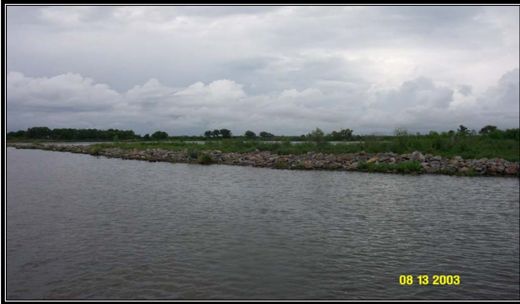
Breach 1 thru 4 – rock dike along Bayou Decade looking north.
