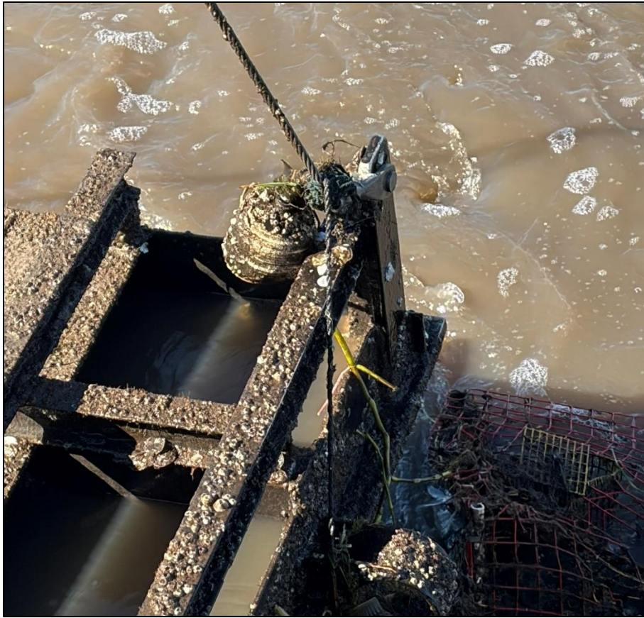
2c. Gate No. 2 – Lifting eye, shackle and cable - North side of Gate
