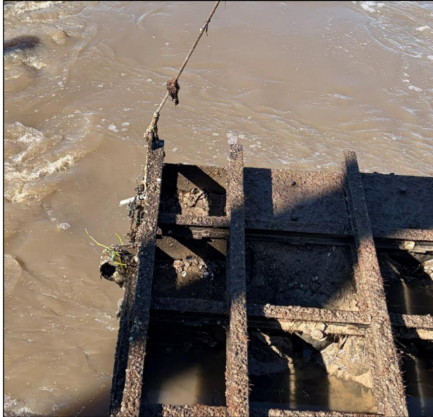
1e. Gate No. 1 – Lifting eye, shackle and cable - South side of Gate
