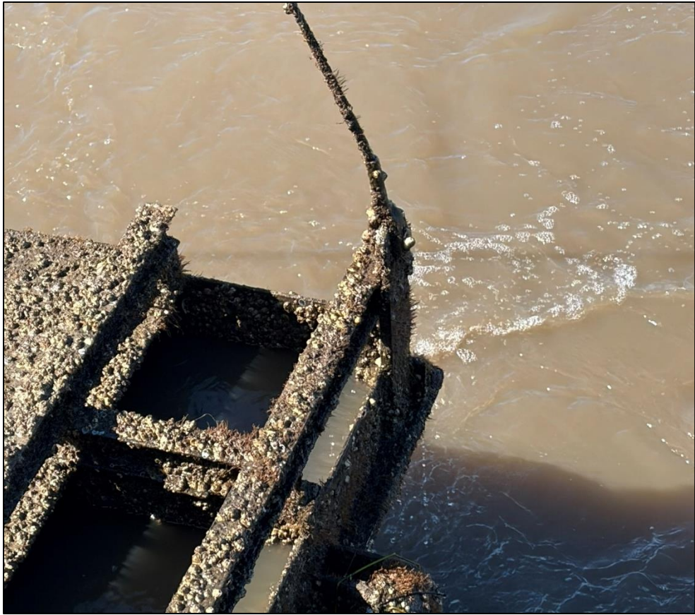
5c. Gate No. 5 – Lifting eye, shackle and cable - North side of Gate
