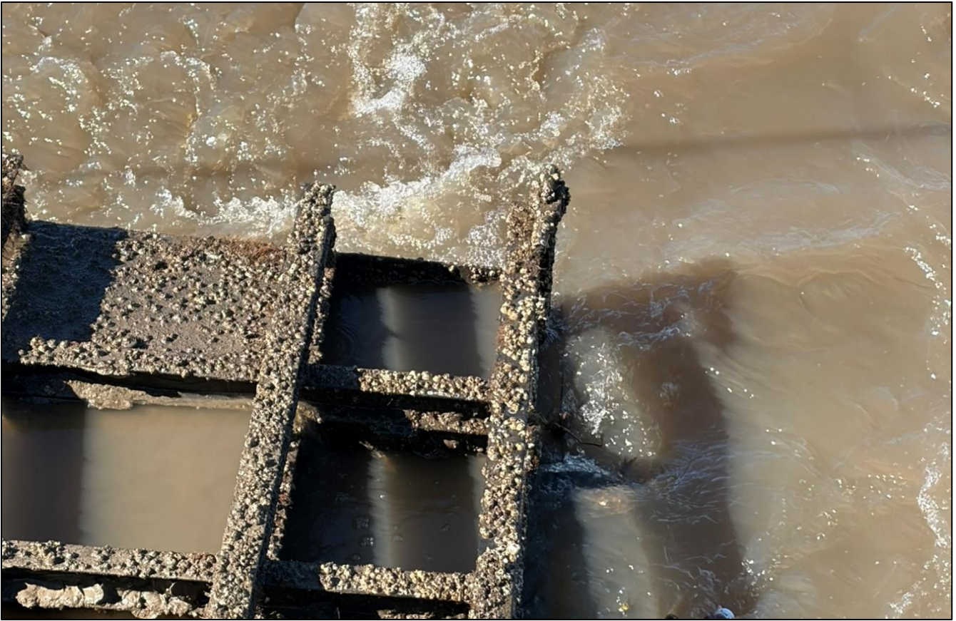
7c. Gate No. 7 – Lifting eye, shackle and cable - North side of Gate. Broken Cable
