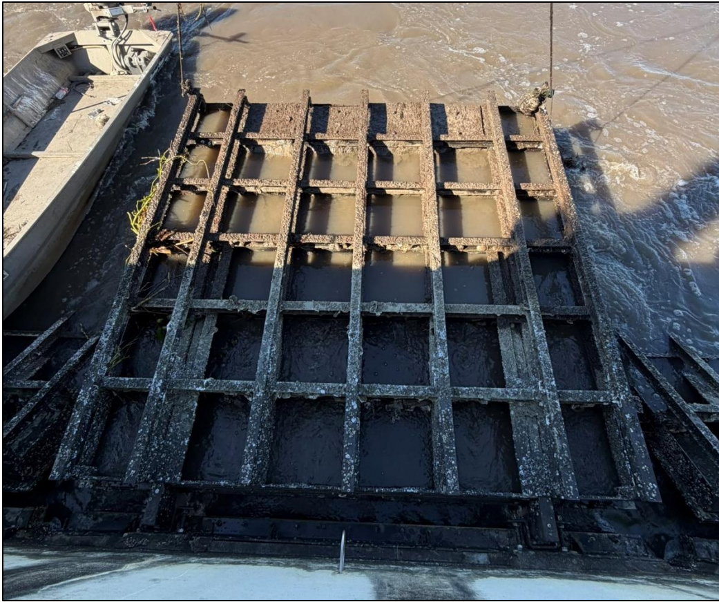
2a. Gate No. 2 – Top View
