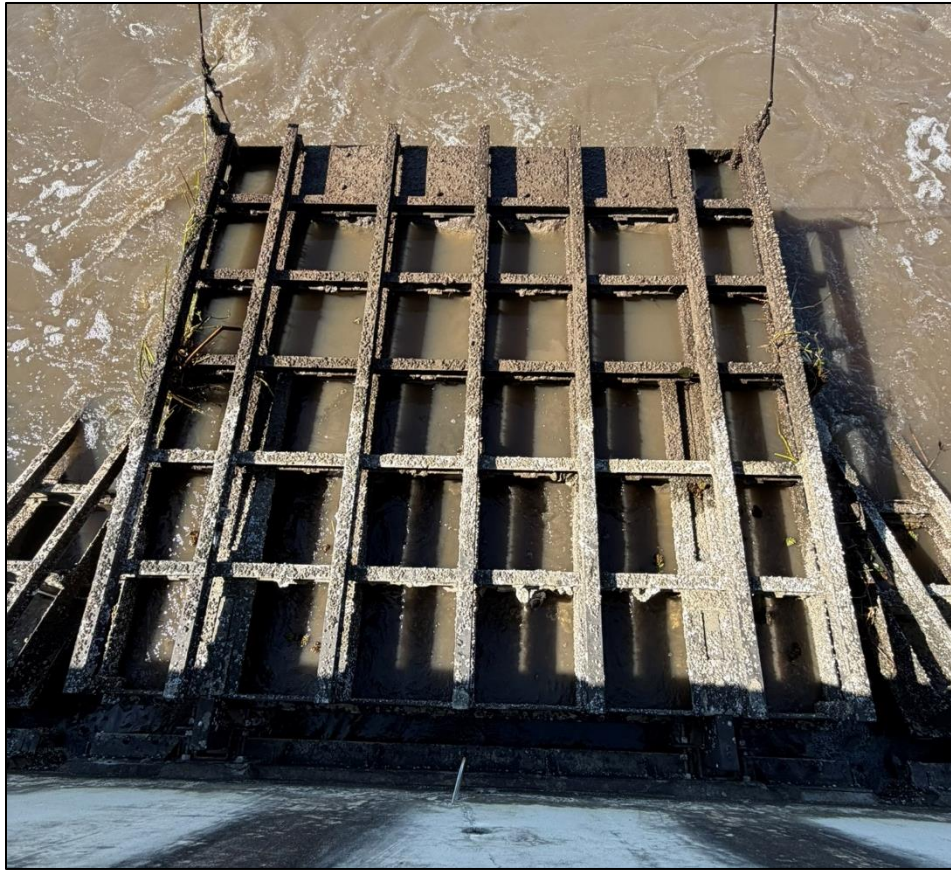
8a. Gate No. 8 – Top View
