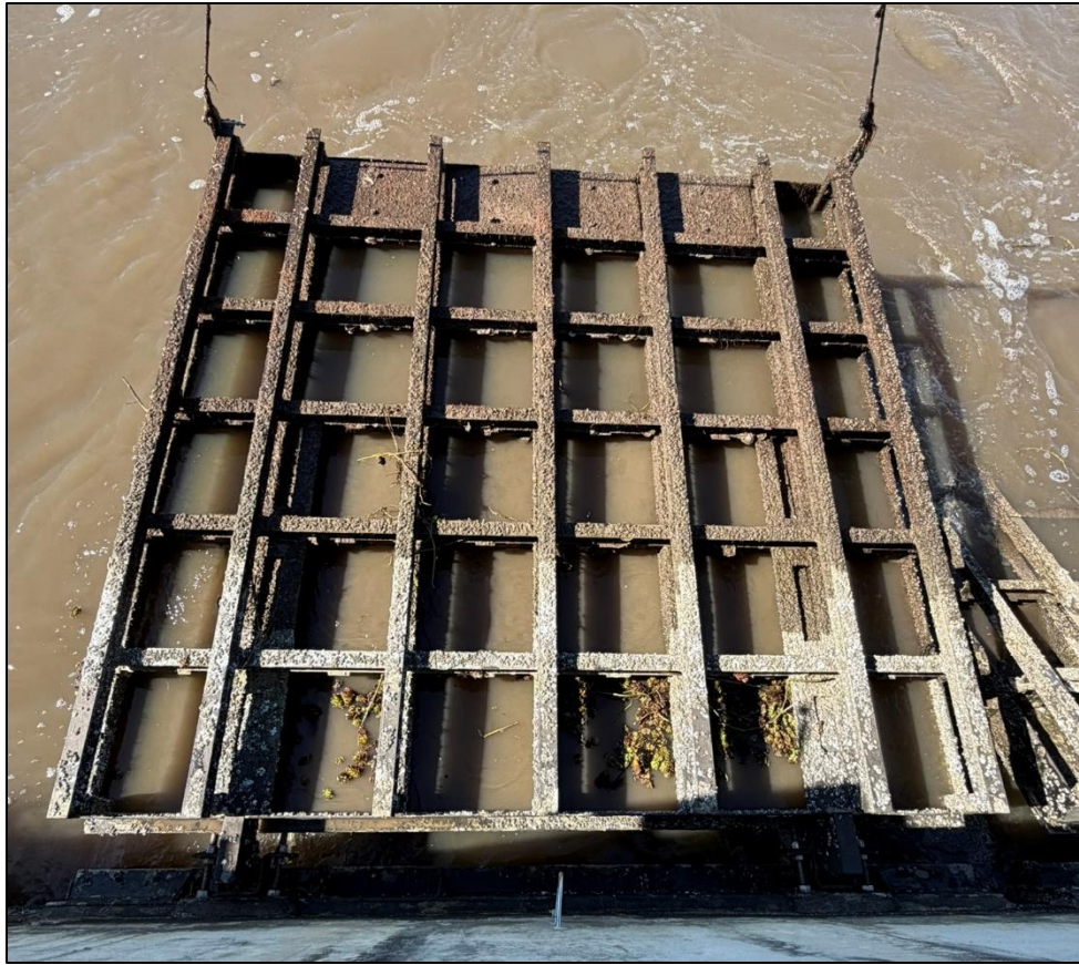
10a. Gate No. 10 – Top View
