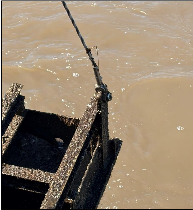
9c. Gate No. 9 – Lifting eye, shackle and cable - North side of Gate.
