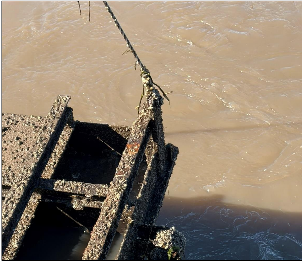
4c. Gate No. 4 – Lifting eye, shackle and cable - North side of Gate
