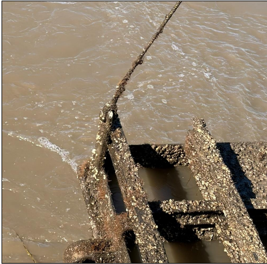
5e. Gate No. 5 – Lifting eye, shackle and cable - South side of Gate
