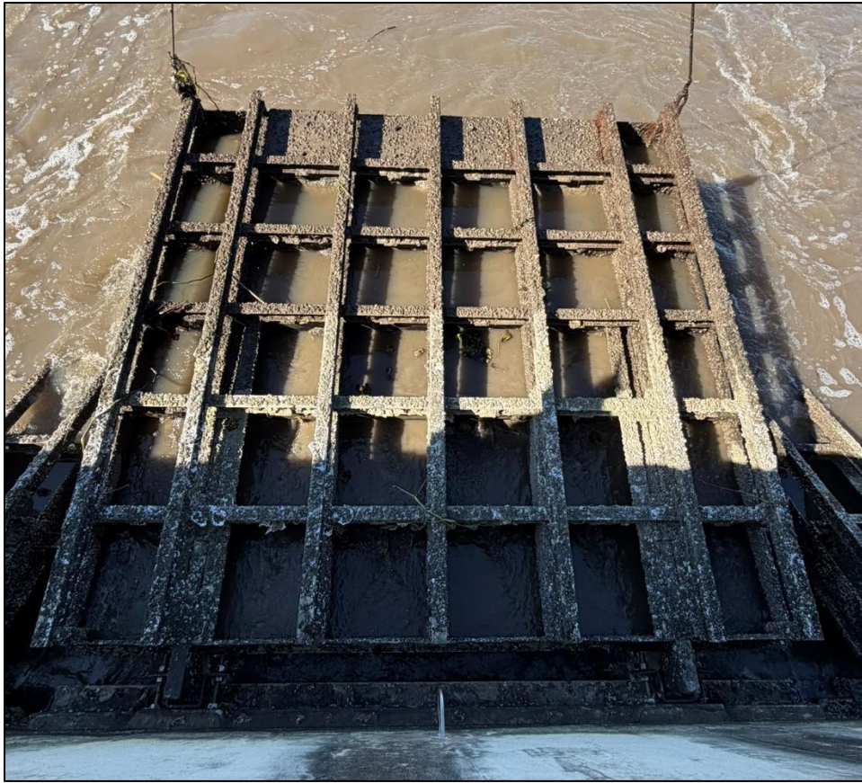
6a. Gate No. 6 – Top View
