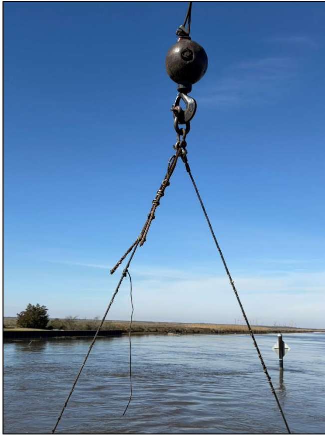
6e. Gate No. 6 – Old, Damaged Lifting cable. (South Cable)
