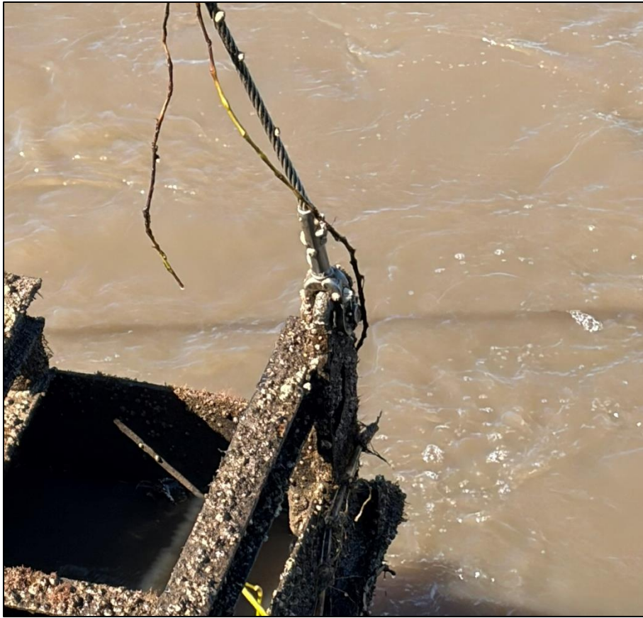
3c. Gate No. 3 – Lifting eye, shackle and cable - North side of Gate
