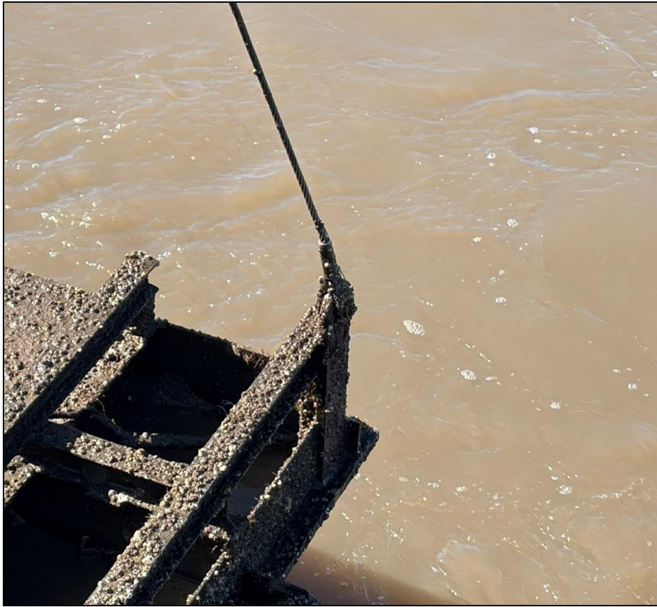
8c. Gate No. 8 – Lifting eye, shackle and cable - North side of Gate.
