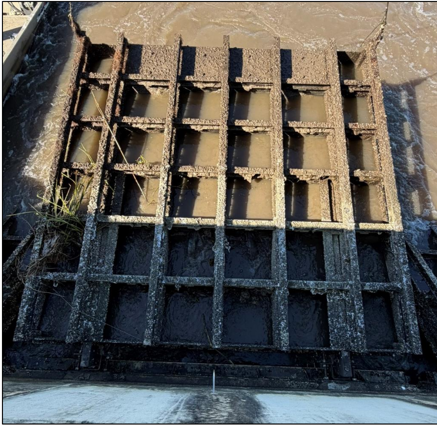
4a. Gate No. 4 – Top View
