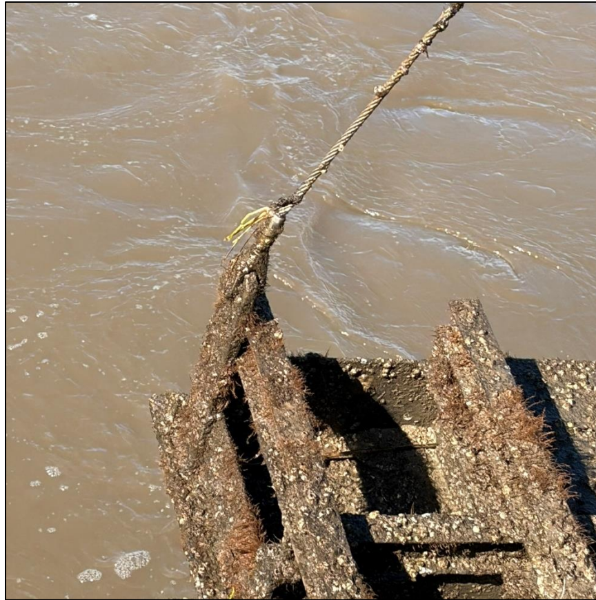
4e. Gate No. 4 – Lifting eye, shackle and cable - South side of Gate
