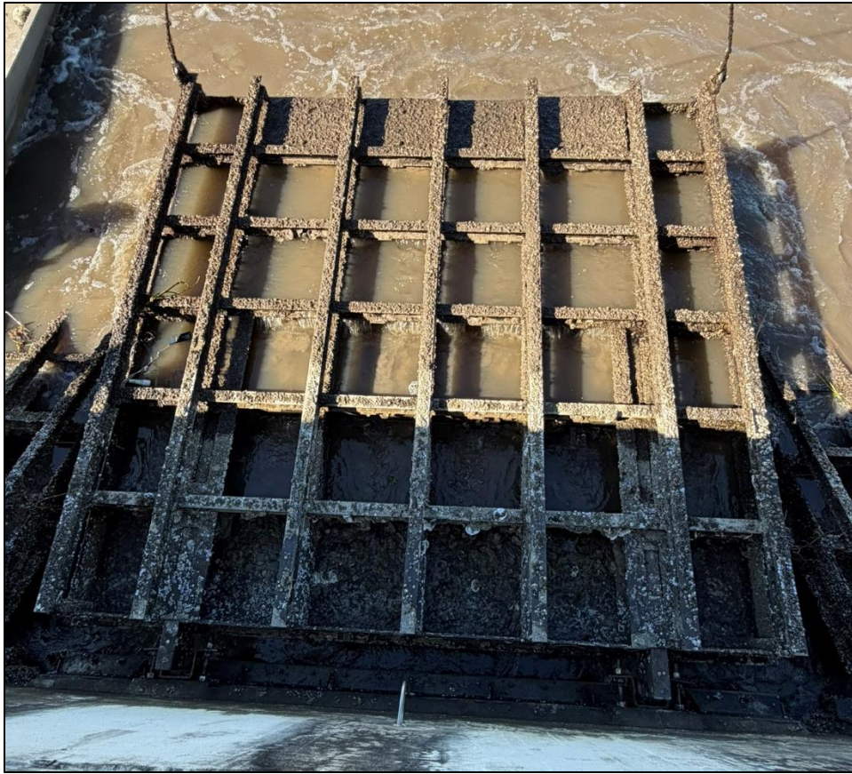
5a. Gate No. 5 – Top View
