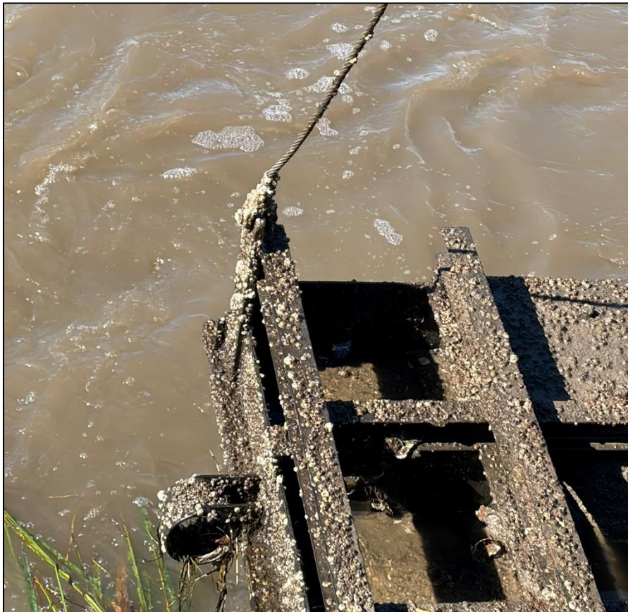
7f. Gate No. 7 – Lifting eye, shackle and cable - South side of Gate
