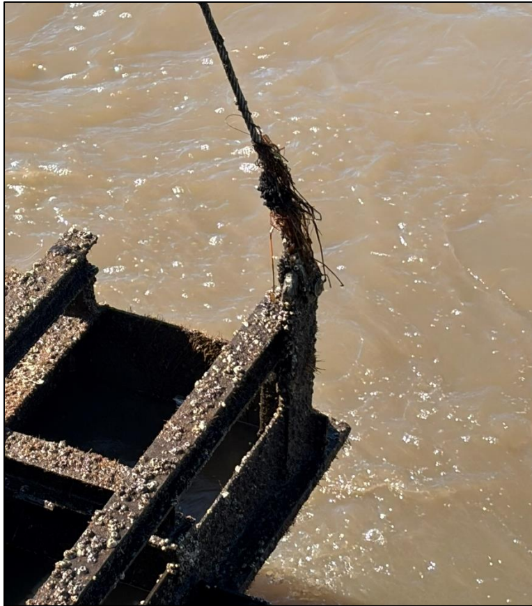
10c. Gate No. 10 – Lifting eye, shackle and cable - North side of Gate.
