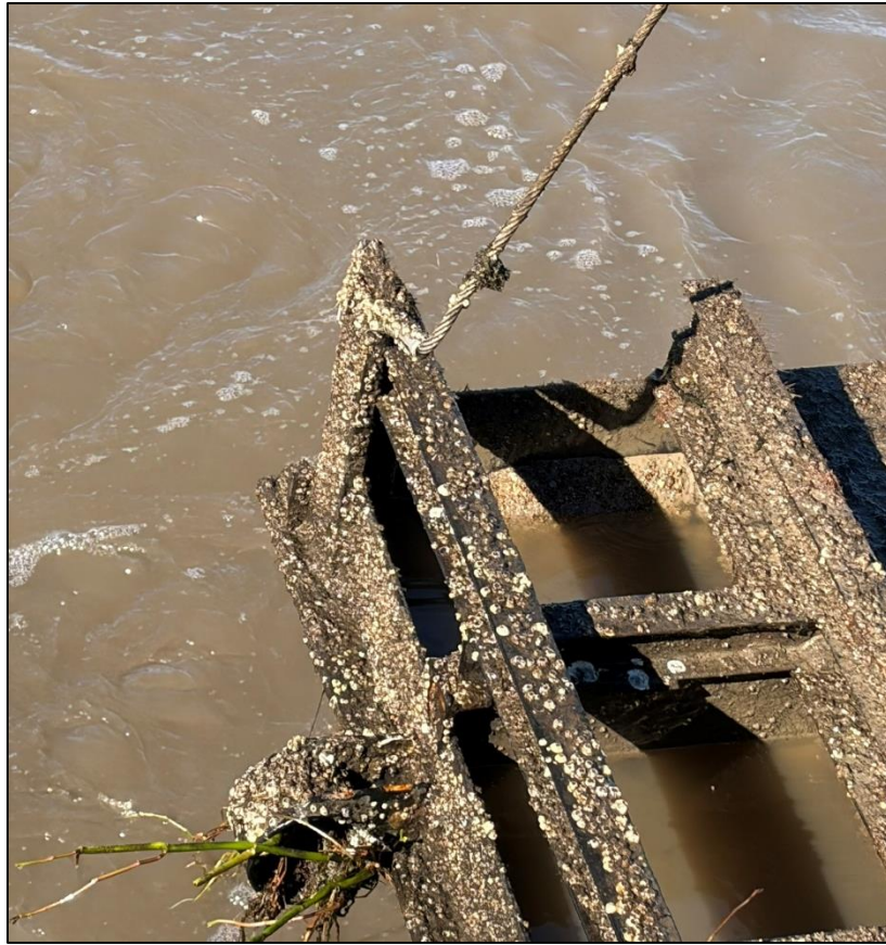
2e. Gate No. 2 – Lifting eye, shackle and cable - South side of Gate
