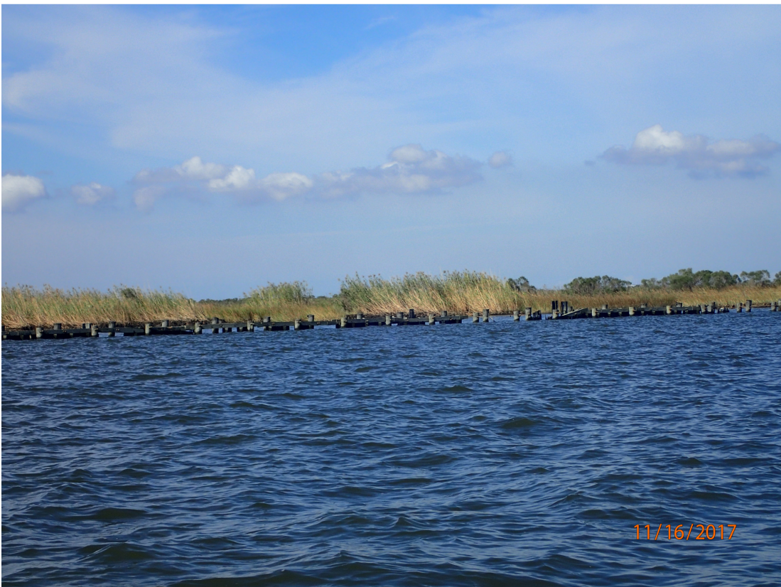
Photo 2: Reach 1 - Damaged Sheetpile Wall
