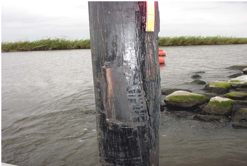
Photograph. 1 – Bayou Dupont Canal Weir. Damaged pile at right side of boat bay as one enters the Pen from Barataria Waterway. Pile was damaged by boat collision during construction. Pile may eventually need to be replaced or reinforced.
