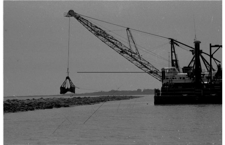
The proposed terraces at Four Mile Canal will be constructed in a similar fashion as shown above. The above photo is of the Captain Buford Berry constructing terraces at the project at Little Vermilion Bay (TV-12).
