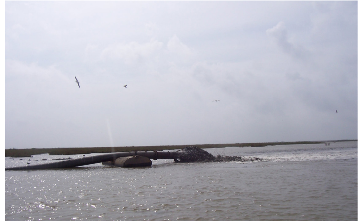
This dredge pipe is rebuilding marsh by depositing sediment dredged from a nearby borrow area. The placed sediment will reach an elevation conducive for growing and sustaining marsh vegetation.
